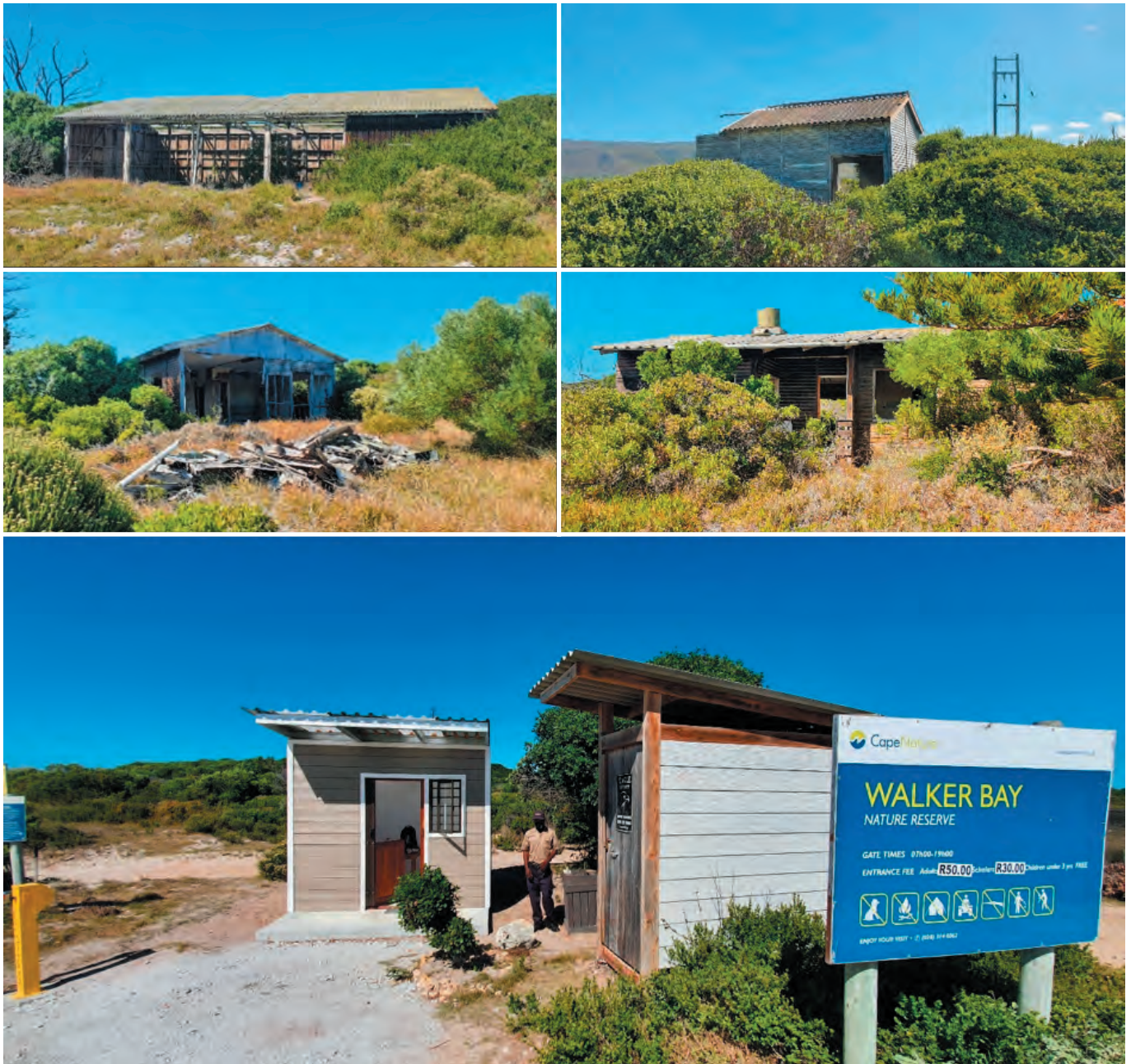
Figure 7.4: The various old, dilapidated buildings (top), the renovated gatehouse, and newly constructed eco-toilet within Uilkraalsmond (bottom). Photos: D. Burger.
