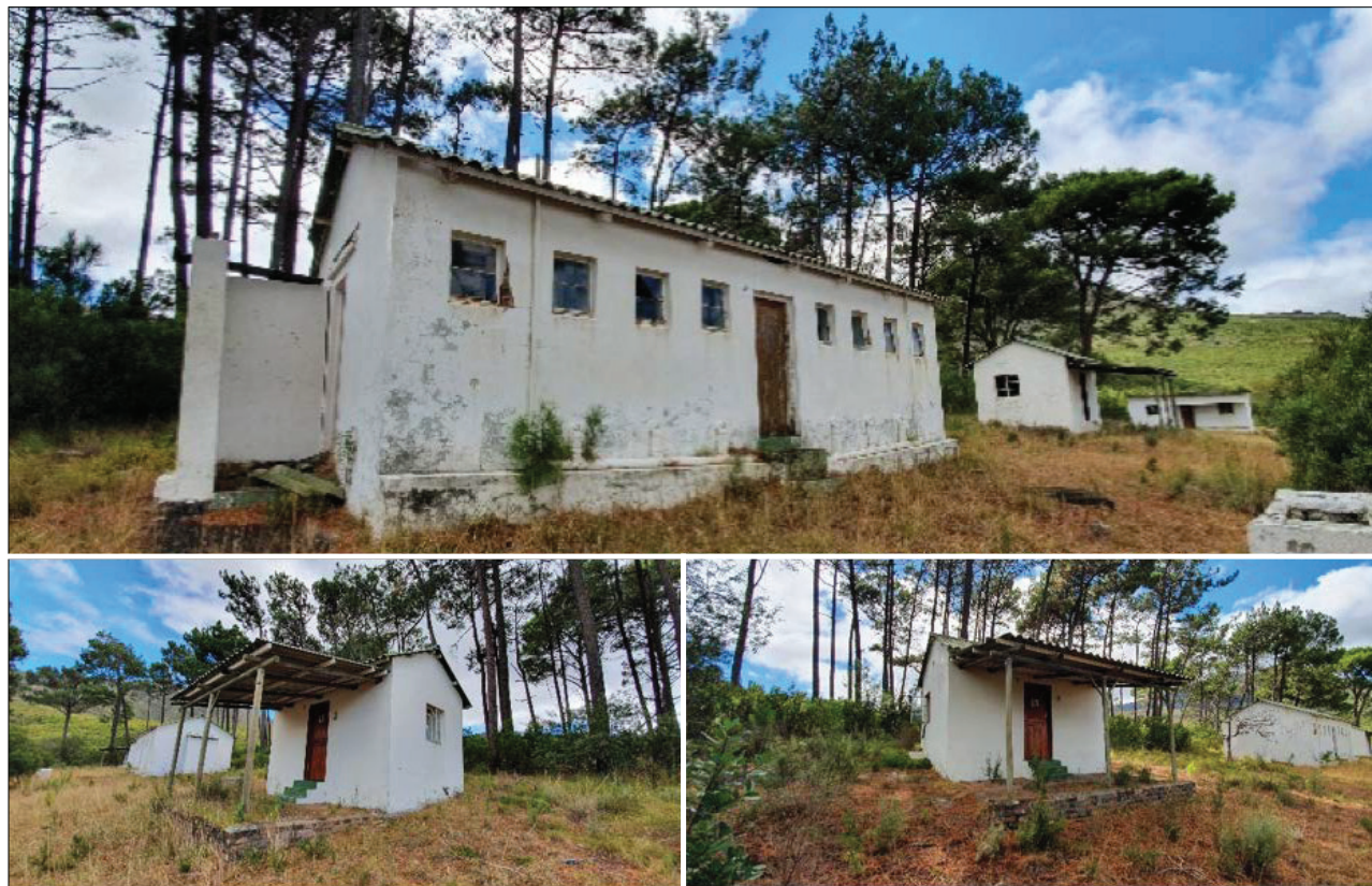
Figure 7.5: The two units and ablution facilities located on Salmonsdam within the Walker Bay Complex. Photos: D. Burger.
