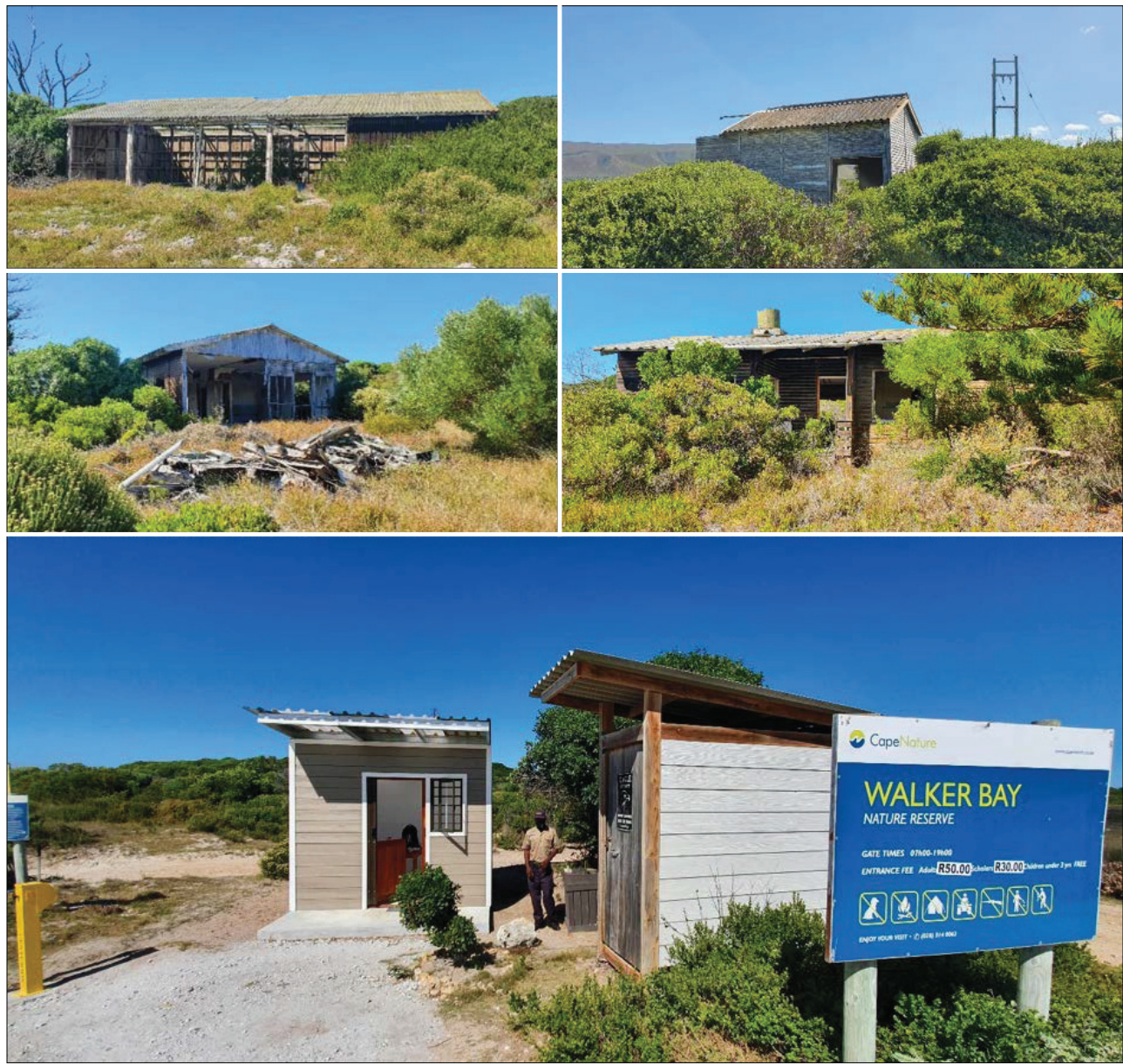
Figure 7.4: The various old, dilapidated buildings (top), the renovated gatehouse, and newly constructed eco-toilet within Uilkraalsmond (bottom). Photos: D. Burger.
