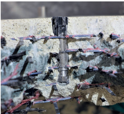
Figure 13: Carbon concrete slab, variant new construction with concrete B2 Hf modified and carbonated, after 14 months free weathering after cutting; the shown A4 heavy duty anchor and all other stainless steel components in contact with carbon are not corroded | photo: Jürgen Triebert
