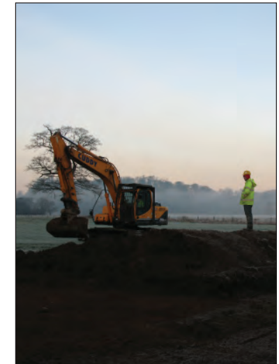
Illus. 3 - Topsoil was stripped from the site using earth-moving machinery under archaeological supervision, in accordance with accepted best-practice.
