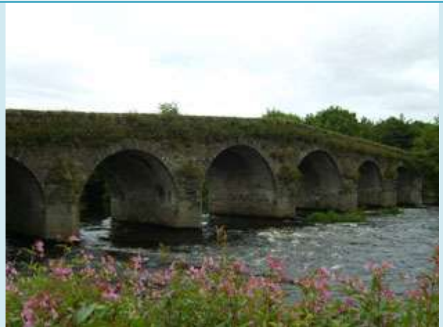
TOWNLAND SCARAWALSH RIVER SLANEY SCARAWALSH BRIDGE, SCARAWALSH NIAH 15702002- now disused- vulnerability increased
