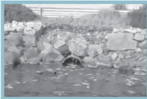
Undersized culverts significantly reduce tidal flow into marsh systems.
