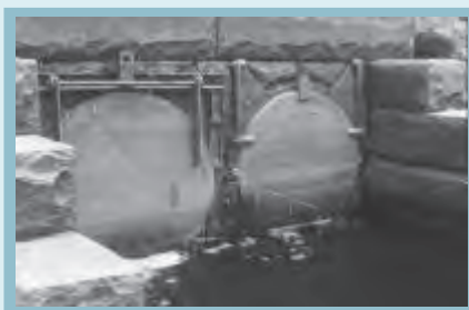
Tidegates deprive salt marshes of essential tidal flow. These gates, on Back River Creek, Woolwich, ME have been removed.
