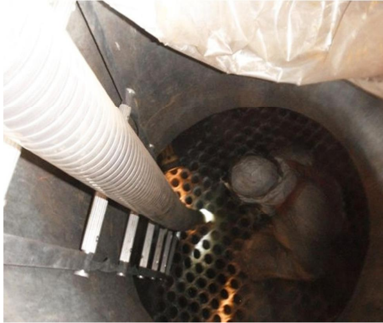
Figure 18: Loading of a tube reactor from the top. The flexible duct is the vacuum system for dust removal.
