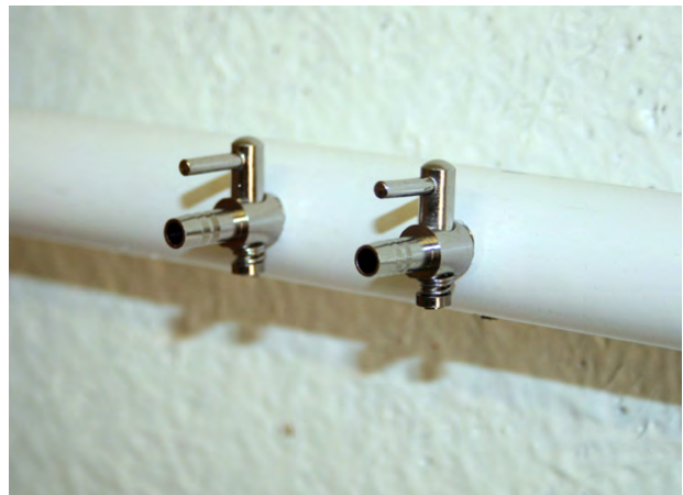
Tidy air supply fed from blower
