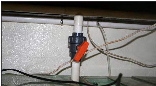
Centralised tanks fed from stop taps
