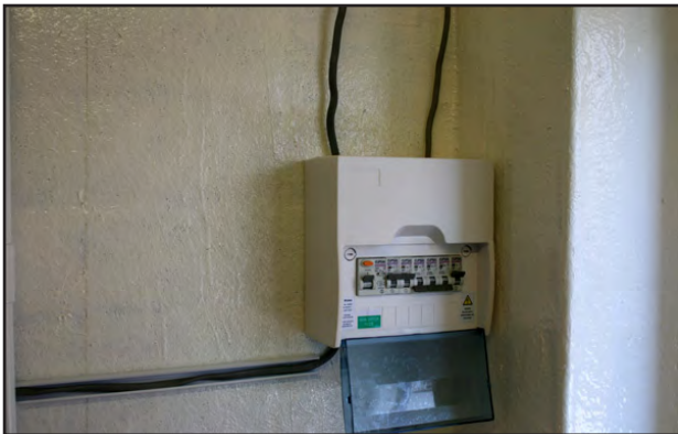
Isolated electrical supply to new fish house
