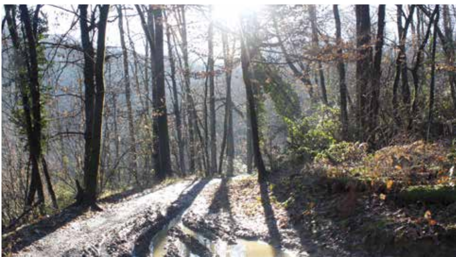
The aqueduct of Via dei Vasi begins at the fountain in Via Ramera and follows a long route through the woods to reach the village of Gallina.
