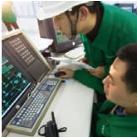
Employees in the control room of the Chongqing cement plant, China
