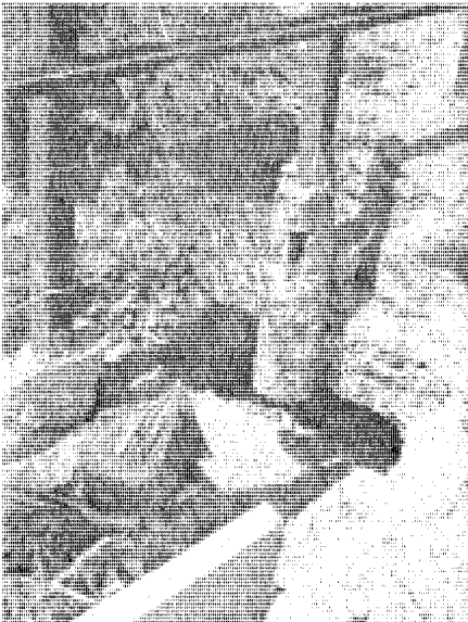
Photo 2: Erosion around a vehicle barrier post during one high water flow event, Organ Pipe Cactus National Monument 2005.
