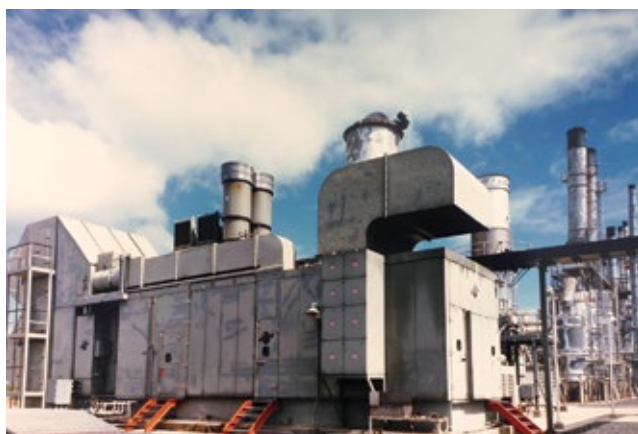
4. Stewart & Stevenson's first LM2500 package was installed at the Hawaiian Independent Refinery in 1983. Photo was taken years later
