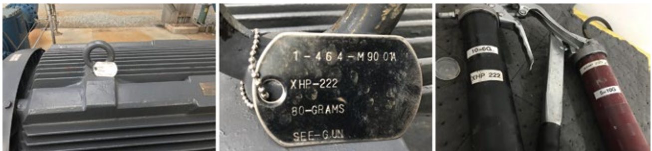
2. Tags made by plant personnel give the equipment number and type and amount of grease required
