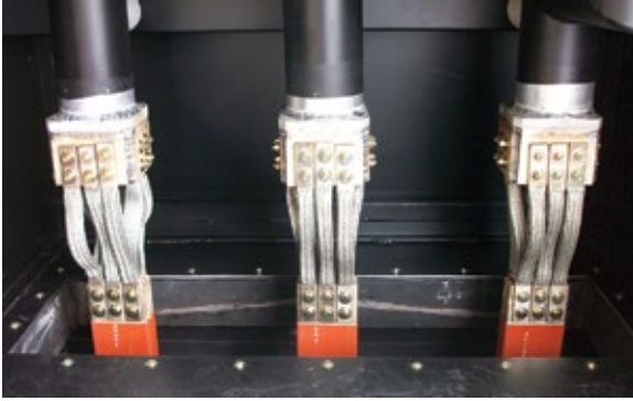
18. Every few years, O&M personnel should verify flex-braided bolted joints are tight
