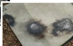
2, 3. Burned insulator boots (left) and damaged duct cover (below) at the fault location
