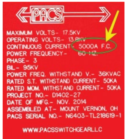
21. Nameplate for generator main breaker reveals F.C.—for forced cooling—after the continuous current rating of 5000 amps
