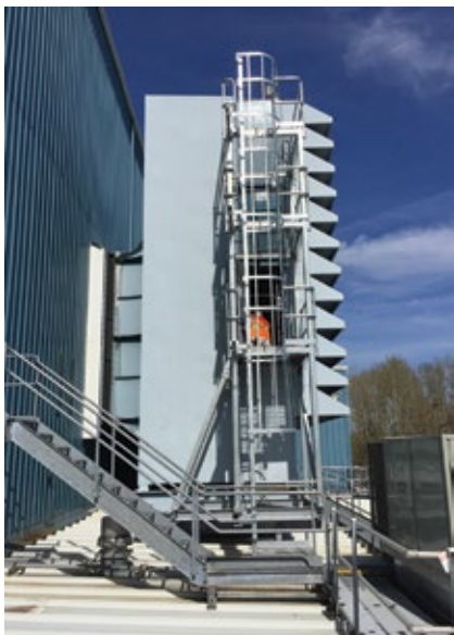
3. Emergency escape tower has landings on each floor of the filter house, making it easily accessible through the doorways installed
