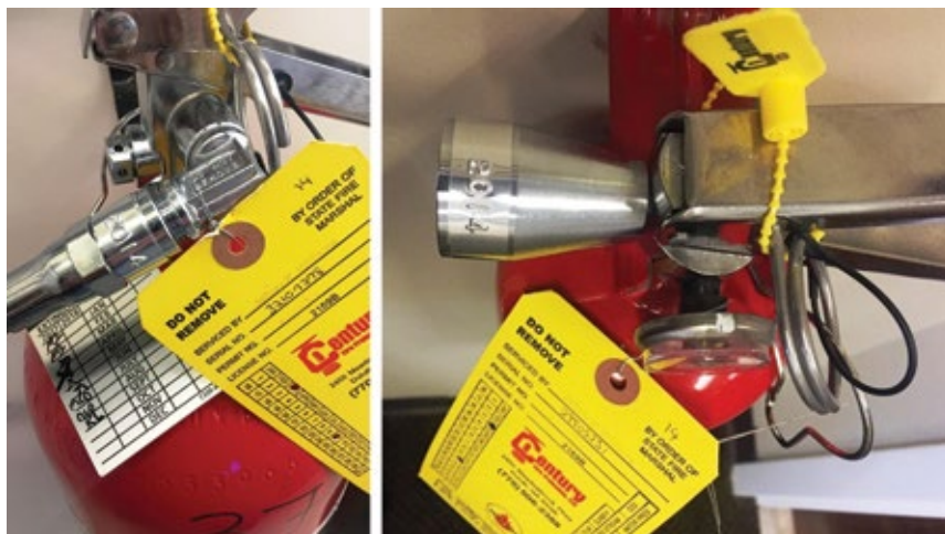
3. Clear labeling of date of manufacture on fire extinguishers is important
