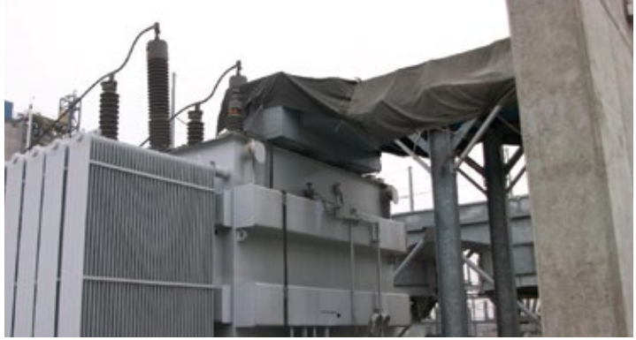
19. Tarps are not reliable leak prevention gear
