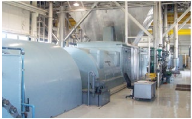
2. Wolverine Power Supply Co-op's STAG 105 looks almost new after 50 years of service
