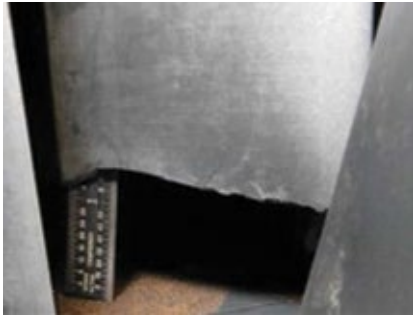
3. Tip was liberated from this S1 vane. Such potential damage is not addressed in either TIL 1884 or 1980
