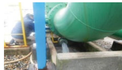
6. Open drain line confirms when heat exchanger is empty
