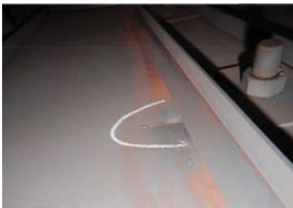
6. Fatigue cracks found in Type-409 liner plate
