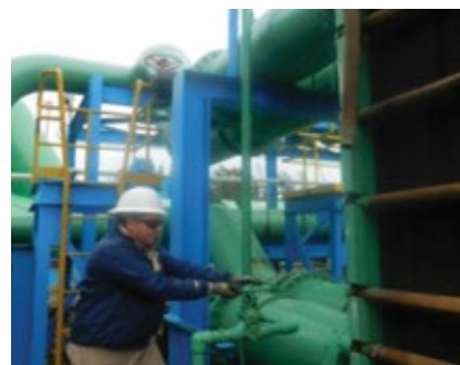
8. Opening the vent valve in the closed-circuit water system is an important step
