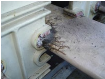
17. Mechanical rubbing of insulation at “choke points” leads to wear, tracking, and failure
