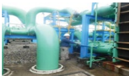
7. Shutting the closed-cycle water inlet valves to the heat exchangers is part of the process
