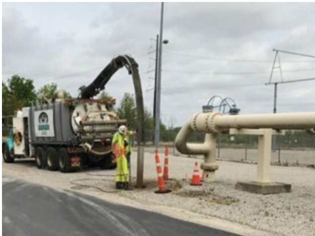
4. Hydrovac system makes holes for bollards with minimal impact to existing infrastructure (left)
