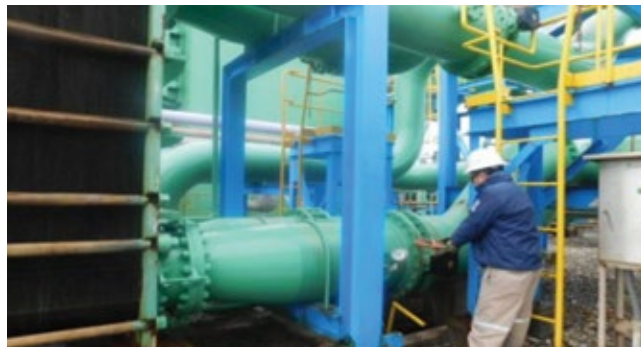
5. Closing the seawater outlet valve
