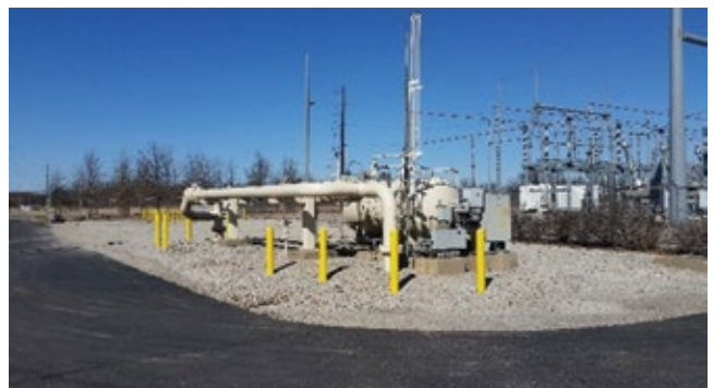
5. Bollards protect gas line at plant entrance (below)
