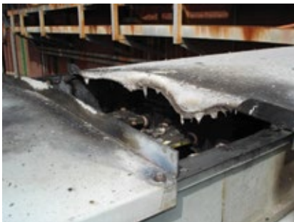
16. Thermal cycling causes bus-duct expansion/contraction conducive to joint degradation, water ingress, and failure
