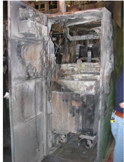
20. 15-kV switchgear overheated and was destroyed by a very hot fire. It vaporized this cubicle as well as a couple of others. Plant was down for 21 days to replace the three cubicles affected, considered a rapid turnaround given project complexity
