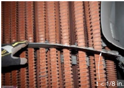
7. Type-304 plate materials downstream of duct burners must be thick enough to prevent damage
