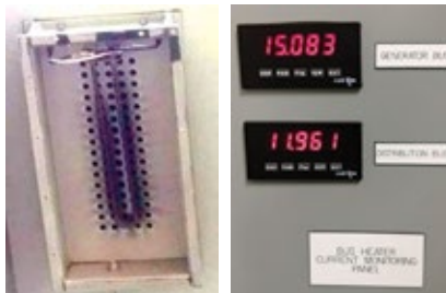
8, 9. Air is injected at each space-heater box located below the bottom bus cover; dry air enters the bus duct through the perforated holes above the heater (left). If any heater circuit trips the current draw will drop by 1 amp (right)
