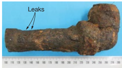
3. LP drum level transmission pipe corrosion (above)
