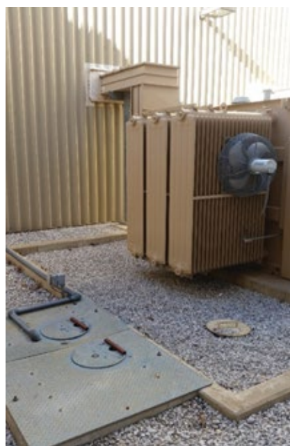
3. Retractable butterfly-valve handles indicate whether valve is open or closed while eliminating a trip hazard
