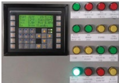
9. PLC-based GEMAC developed by PAL is an option for plant owner/operators that can't justify a full-blown controls upgrade
