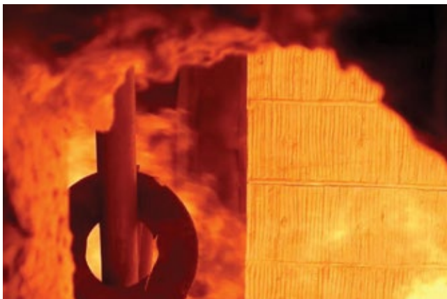
HRST Inc. With the duct burner at maximum firing, use view ports to visually observe the flames for length and shape. Important to avoid flame impingement
