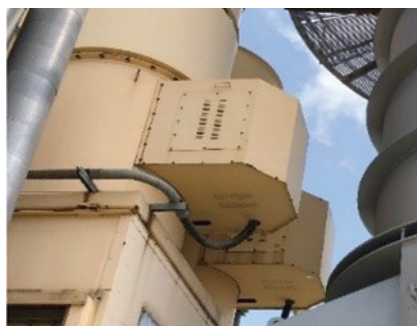
1. Bulky doghouse panels must be removed to do maintenance
