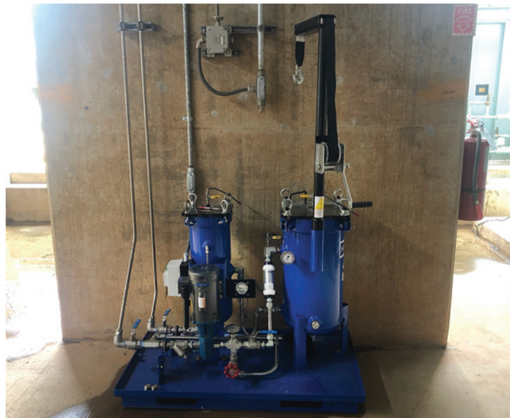
Conditioning skid keeps EHC fluid in good health
