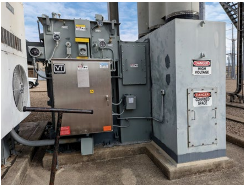
1. Excitation transformer is tied to the isophase bus through a dry bay shroud, where the flashover occurred
