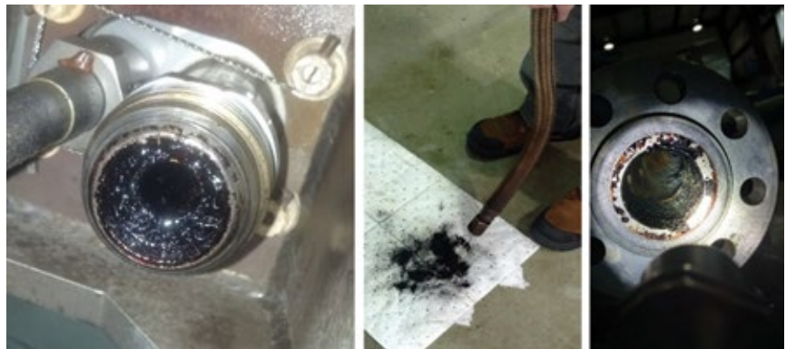
1. Coking in fuel nozzles, gas supply header, and hoses impeded transferring back to gas fuel after operating on distillate oil
