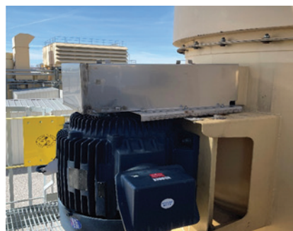
2. Pulley/belt guards benefit safety, improve reliability
