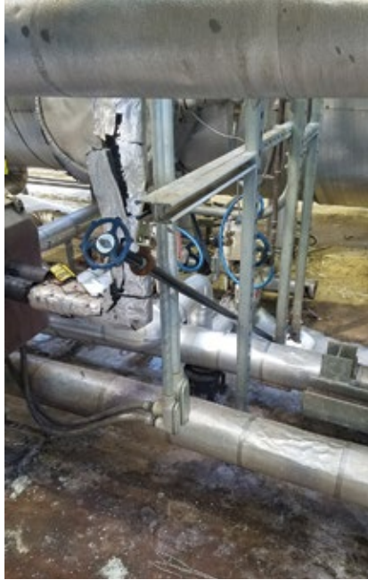
5. Valve operator extension eliminates crawling under piping
