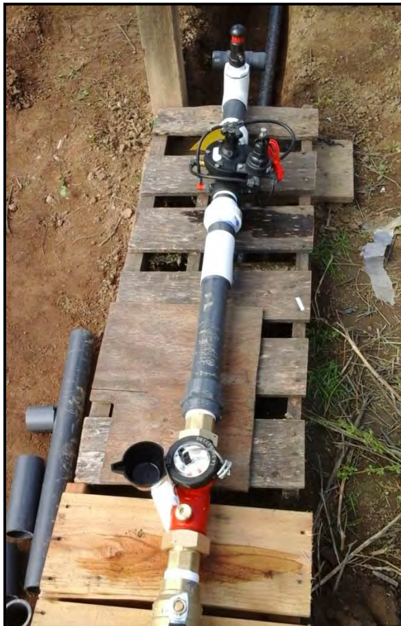
Figure 1. New 2" irrigation mainline with flow meter and adjustable pressure regulator
