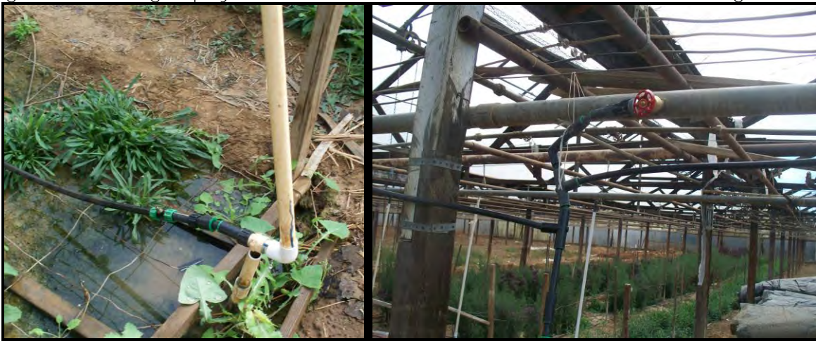
Figure 2. Existing drip system with overhead steel submain and mainline and gate valve
