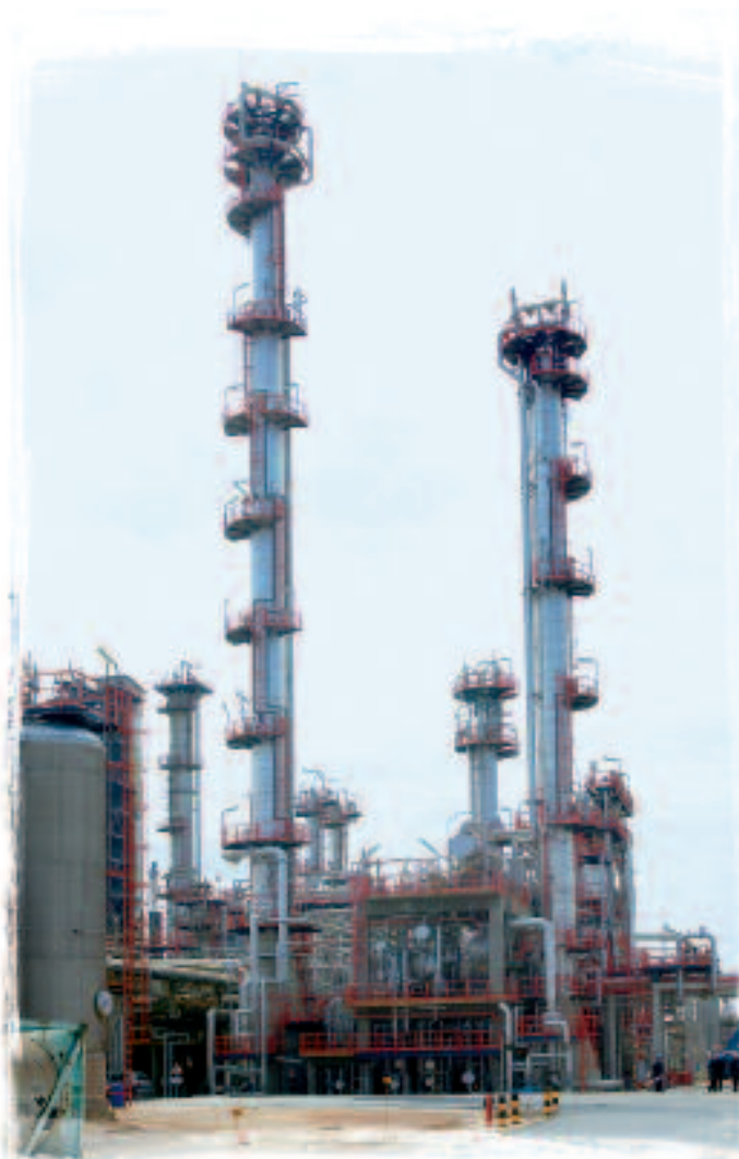
Biofuels plant at the "La Rábida" refinery.
