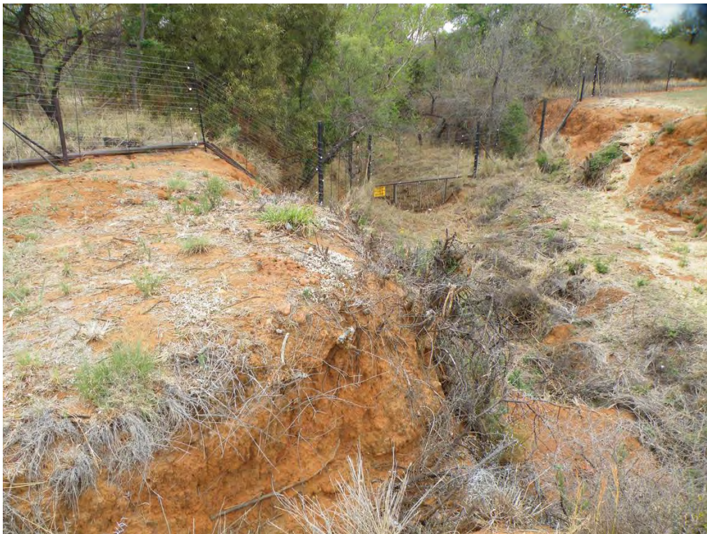
Plate 4: A view a mainstem watercourse, a tributary of the Sleepfontein River, showing a high level of degradation and clearing of any riparian vegetation within road servitude
