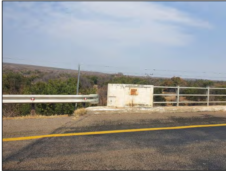
Figure 4-9: View of a bridge along the R516 road in the project area, constructed in 1975.
