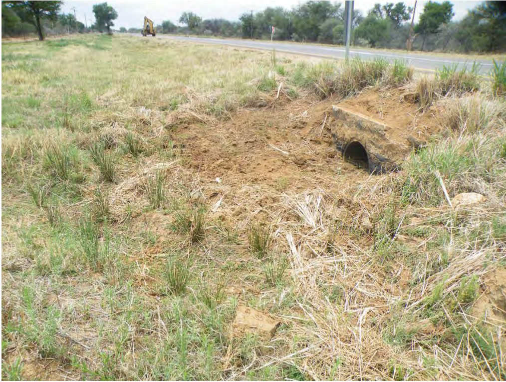
Plate 1: A view of a minor culvert, typically associated with stormwater management and not directly associated with a watercourse or drainage line
