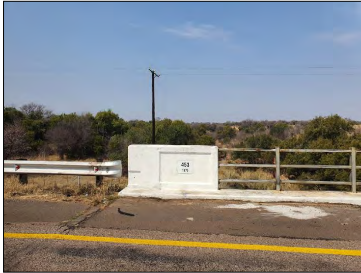
Figure 4-11: View of a bridge along the R516 road in the project area, constructed in 1975..
