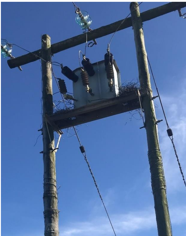
Figure 75: Crow nests constructed entirely out of wire may become a fire hazard.
