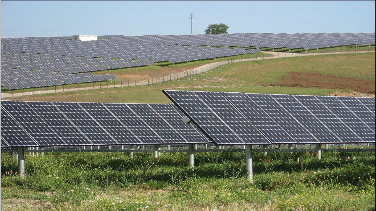
Figure 2-7: A photovoltaic array in Masdar (United Arab Emirates) showing typical concrete “foot” structures.
