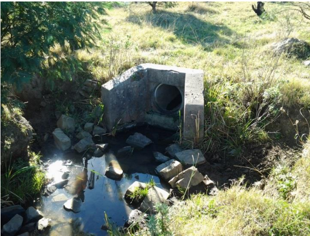
Figure 5.8: The discharge point located below the water reservoir
