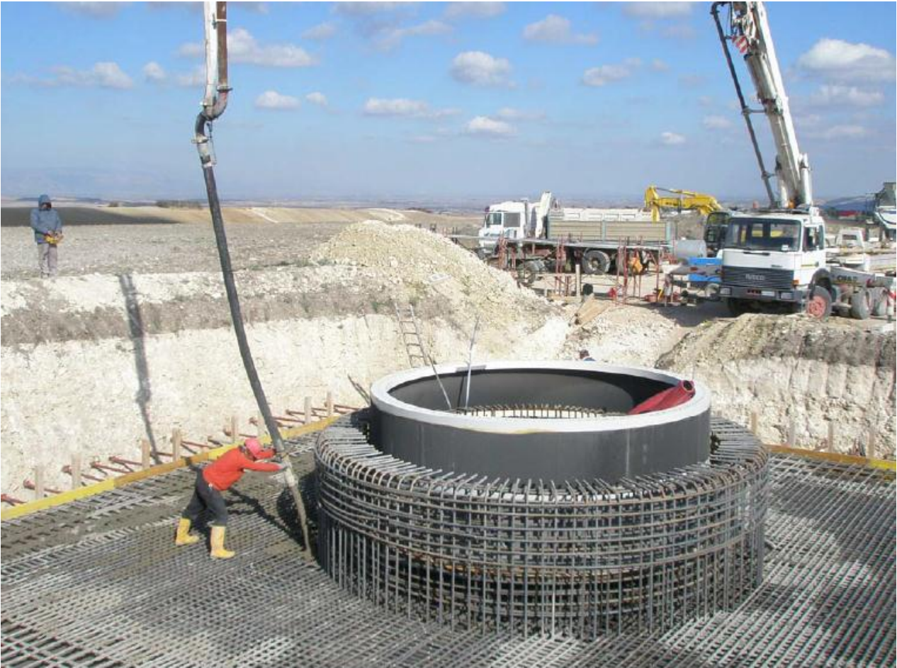
Plate 2-1: Concrete pouring of a turbine foundation – note the tower base collar in the foreground
