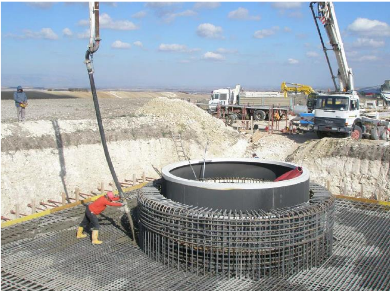
Figure 2-6: Concrete pouring of a turbine foundation – note the tower base collar in the foreground.
