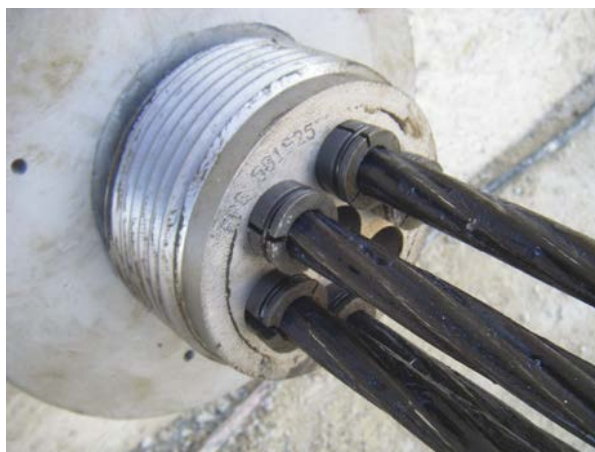
Picture 7.19b: Installation of the anchoring block and wedges prior to stressing (© Soletanche Bachy)
