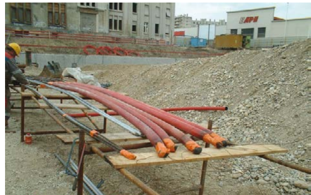
Picture 6.2: Note the sheath of the free part of these ground anchors being assembled on-site (© Sefi Intrafor)
