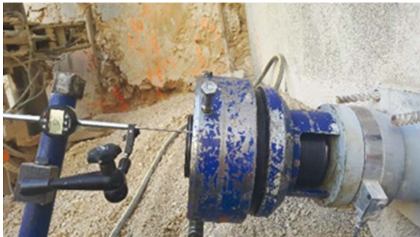
Picture 8.10: lock-off test of a ground anchor with an instrumented head (© Freyssinet)
