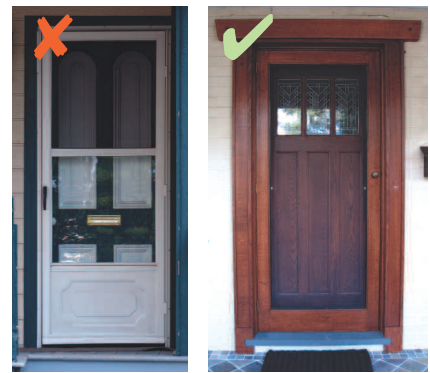
The aluminum screen door on the left hides the details of the historic paneled door behind it, while the screen door on the right highlights the main door. The panel on the right can be replaced with a acrylic panel in winter.
