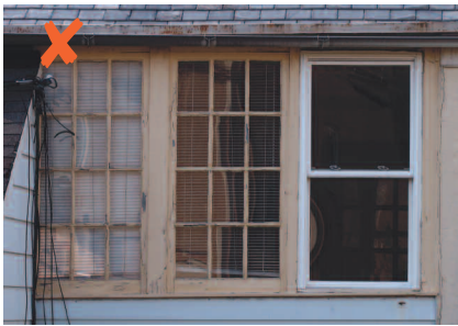
If a window needs to be replaced, the new window should match the original in design and material. The repair above is not appropriate in a historic district.
