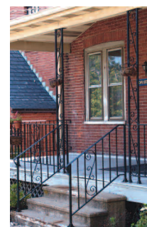
The original columns and balustrades of this porch were replaced with wrought iron; the new posts look too light-weight and visually transparent to support the porch roof.
