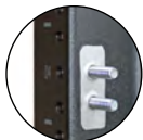
Ground Studs located directly on rack channel
