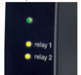
LED operating status indicators
