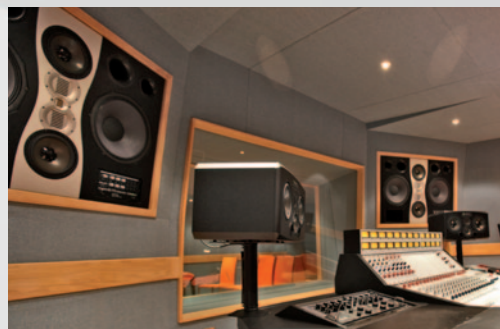
S7A Mk2 & S3X-H Installation "Fayez AlSaeed Sound" Studio, Dubai (UAE)
