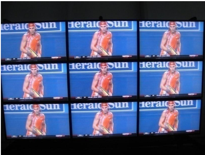
Figure 31. 3x3 Video wall with the same channel playing on each screen
