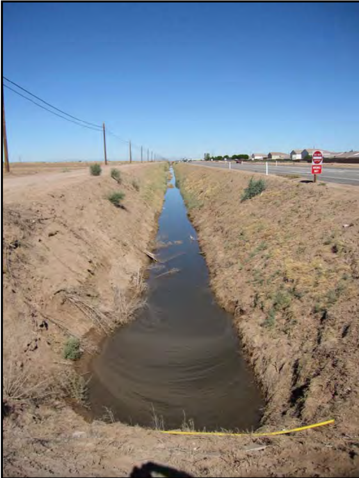
Photograph 1 Looking north along Dahlia Drain. Service road is on the left (west) and SR 86 is on the right (east).
