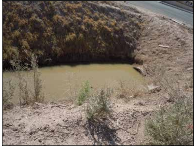
Photo 12. Potential Jurisdictional Area: The drainage pipe in this photograph runs under Neckel Road. Photograph taken facing southeast.
