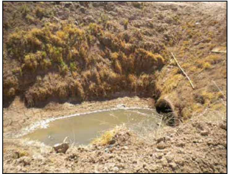
Photo 6. Potential Jurisdictional Area: The drainage pipe in this photograph runs under Neckel Road. Photograph facing southeast.
