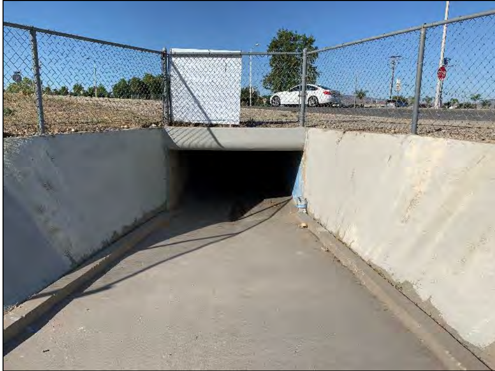
Photo 9. Culvert entrance on east side of Wabash Avenue. Adjacent to the Project site, on the east side.
