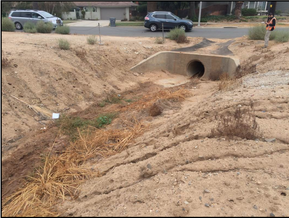
Photo 5. Concrete culvert located underneath Highland Avenue at the northern end of the jurisdictional drainage (facing north).
