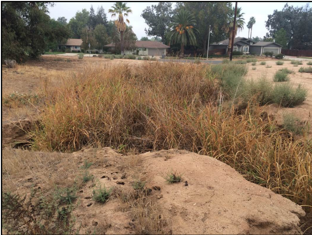
Photo 8. Northern section of jurisdictional drainage near concrete headwall and Highland Avenue (facing north).
