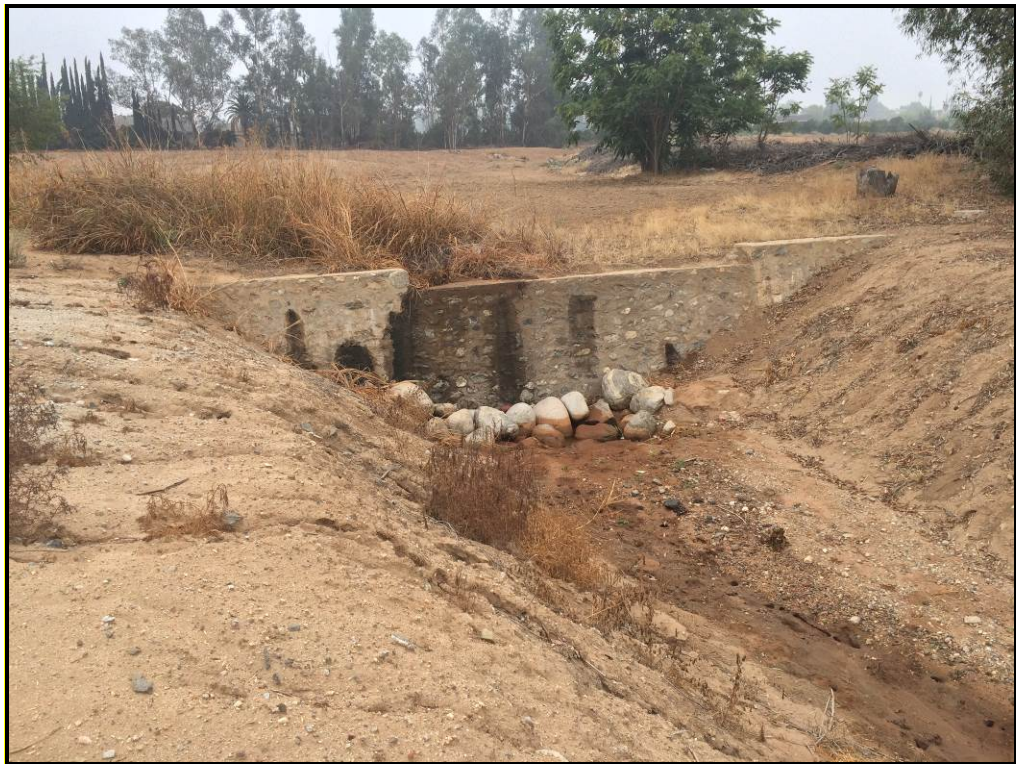
Photo 6. Concrete headwall located between Highland Avenue and the jurisdictional drainage (facing south).
