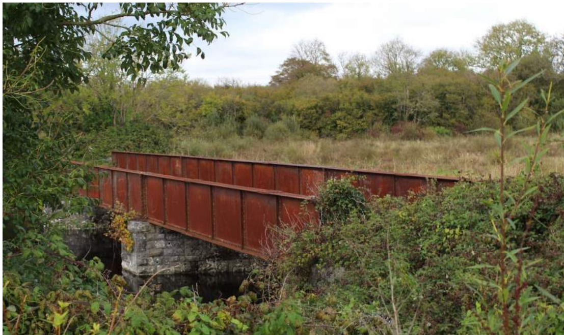
Plate 5-14 Railway bridge over the River Fergus with marginal lands and shrubby vegetation seen from Aughateeroe residential estate
