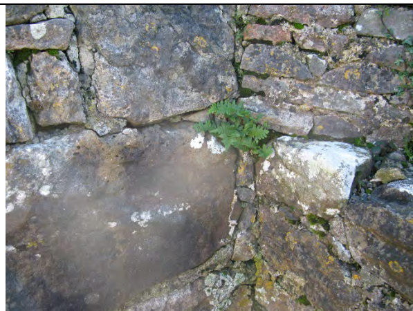
Open joints and fern growth to internal walls at St Brigid's Church.
