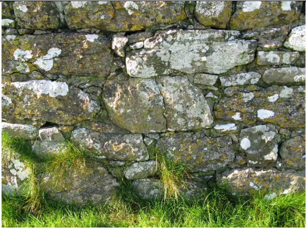
Open joints, grass to joints and cracked stone relating to the use of cementitious mortar.
