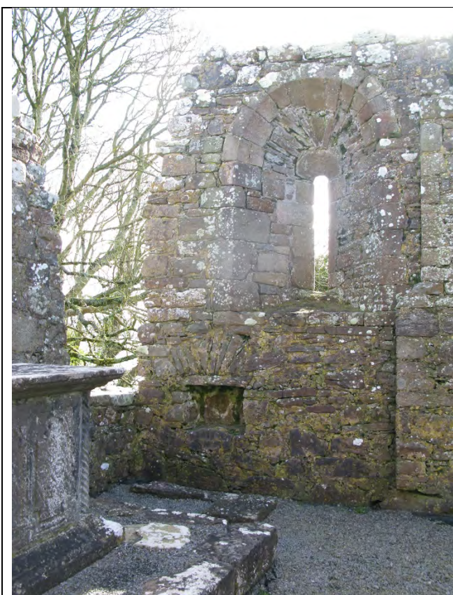
Detail showing splayed window opening to St Mary's Church south wall. Note pilaster rising to right of image.
