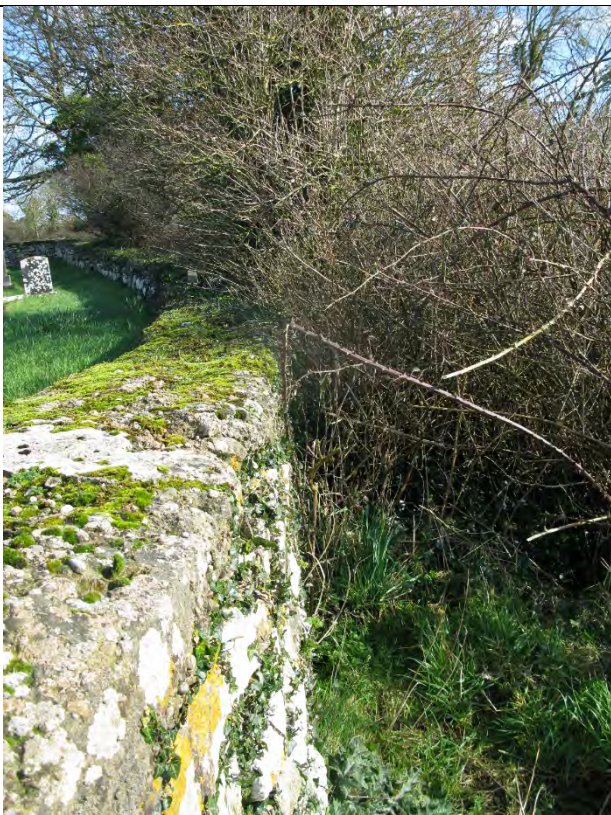
Image showing continuation of south enclosure wall. Not the overgrowth against the external face of the wall along with the moss and ivy growth to the top and side.
