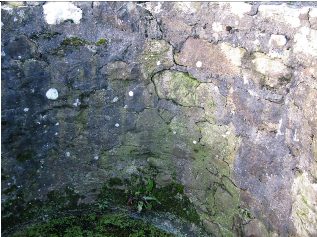
Note cracking along mortar joints to internal wall of well. Wall would appear to have been pointed with cementitious mortar.
