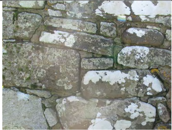
Detail showing loss of bond between stone and cementitious pointing.
