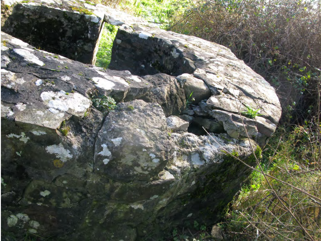
Image detail showing loss of stone to the well wall.
