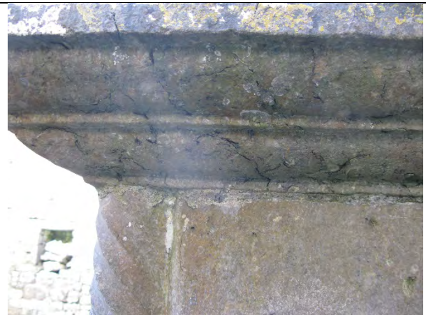
Image showing cracking and crazing to stone.
