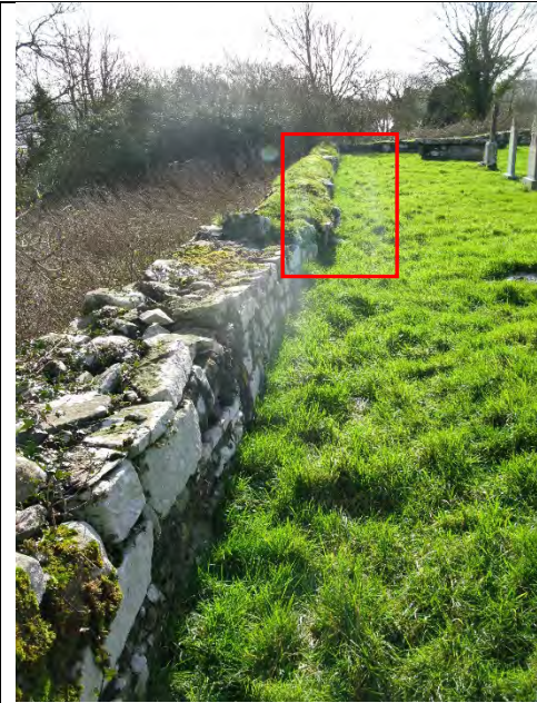
Image showing eastern wall to Saint's graveyard with decayed flashing and vegetative growth. Bulge in wall indicated by red highlight.
