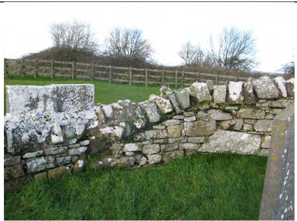
Wall to north was it slopes to meet the church wall. Note dislodged stone.
