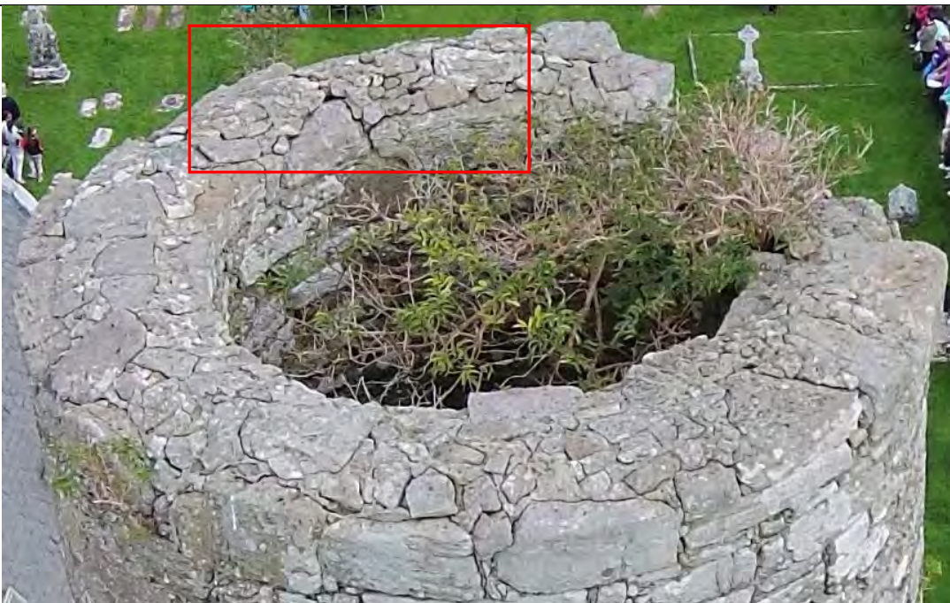
Note poor condition of the stone flaunching to the tower top.
