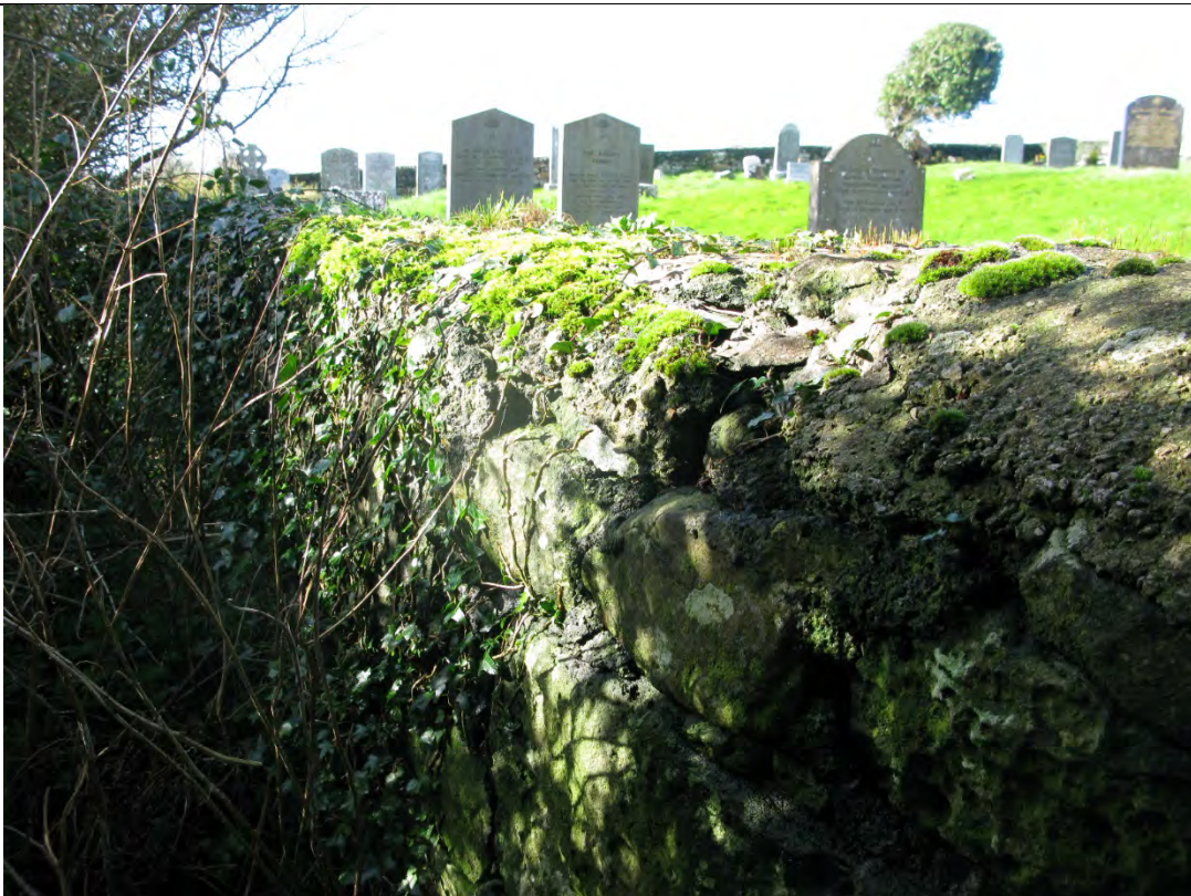
Image showing south enclosure wall. Note vegetation and failed flashing.
