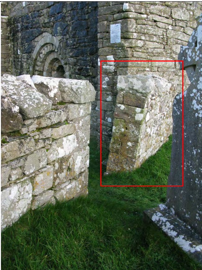
Image showing the leaning wall to the south west of St Caimín's church. Note open joints and vegetation to section of wall to the fore. This section of the wall is present in Robert French's photographic image c.1865
