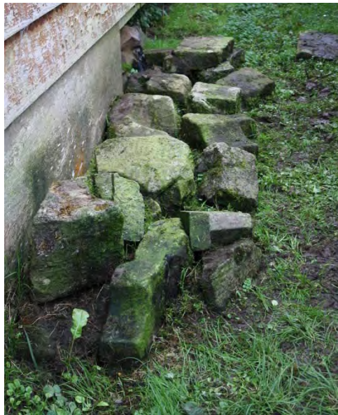
Fig. 84: Loose masonry to north side of OPW shed (Photo: C. O'Leary)
