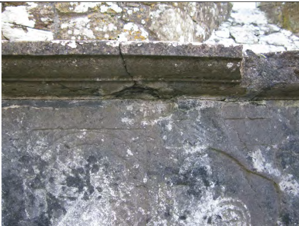
Detail showing chipped and broken stone.
