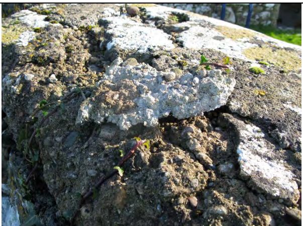
Detail showing cracked flashing and ivy growth.
