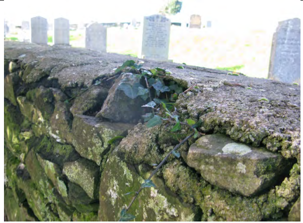
Detail showing failed flashing to wall top with ivy growth.
