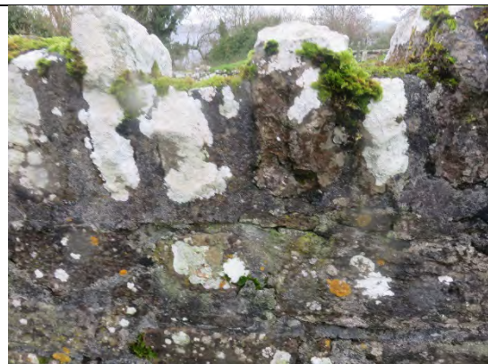
Detail showing cementitious pointing to north outer wall with vegetative growth.
