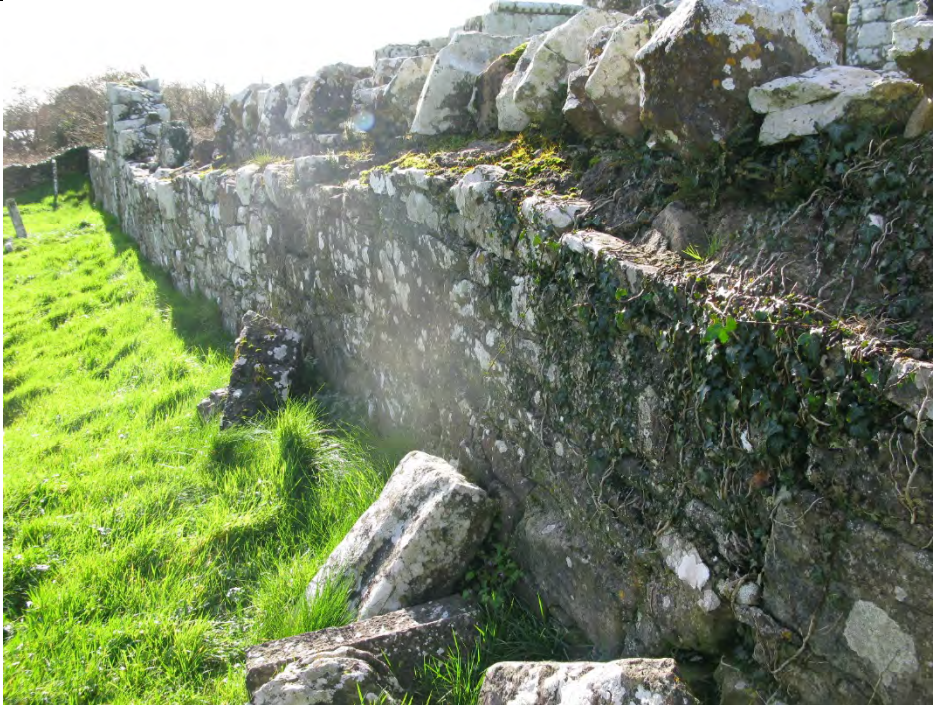
Image detailing exposed ledge and serious leaning to west wall at northern end. Note loose stone to base of the wall and ivy growth.
