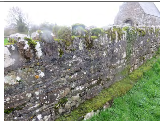
4.4.1.1.1.1 Detail of external north wall showing plinth ledge to base. Not moss growth.
