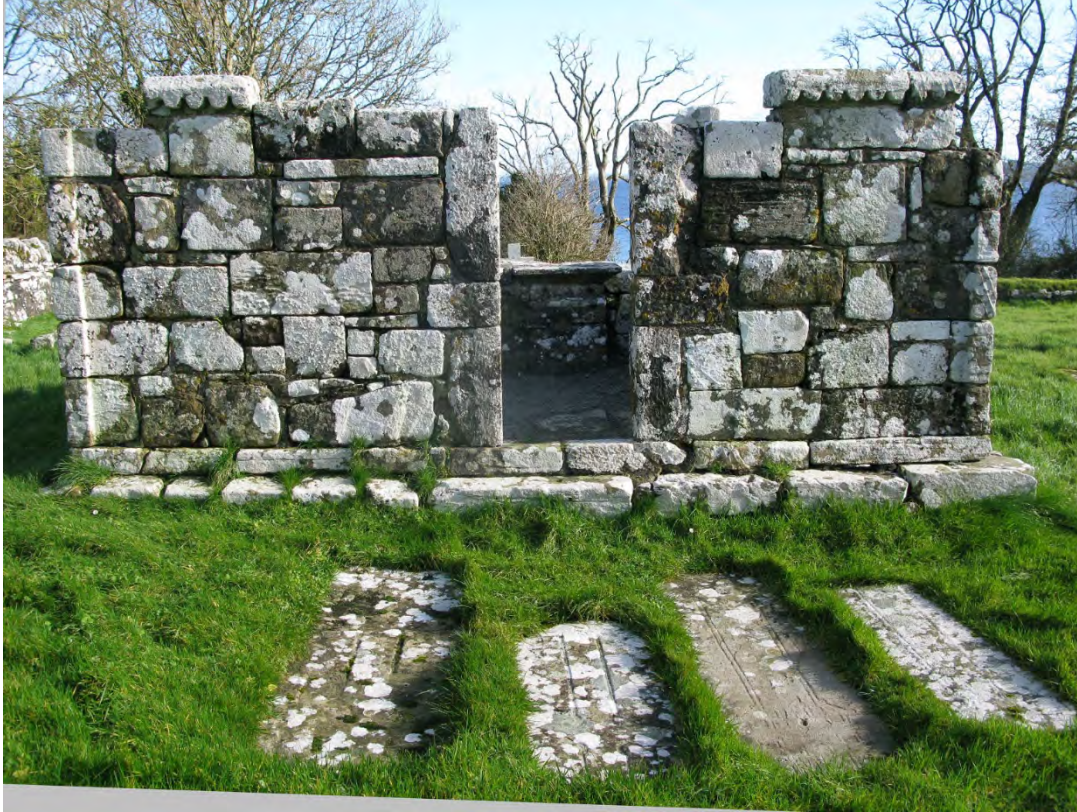
Image showing west elevation to Teampall na bhFear nGonta. Note grass to plinth joints.
