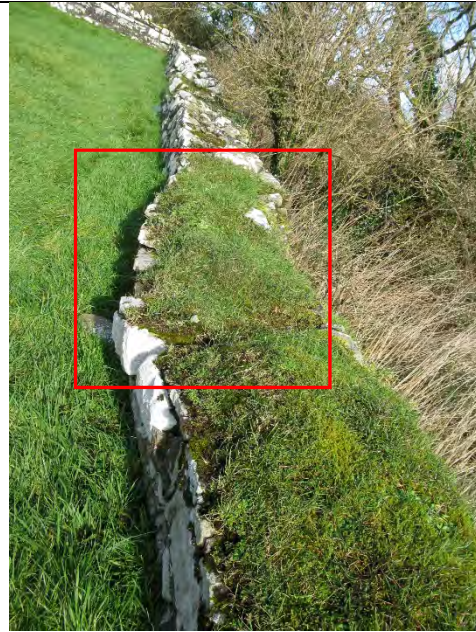
Image showing eastern enclosure to Saint's graveyard. Note the displaced stone and bulge with turf growth to the wall top holding moisture within the wall. Also note extensive vegetation to the outer side of the wall.
