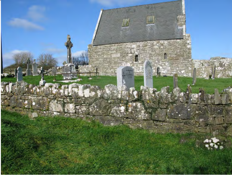
Image showing south wall to enclosed graveyard note ivy growth and loose stone to base of wall.
