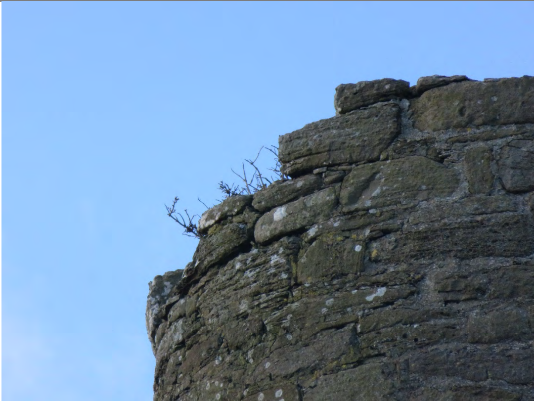
Note tree growth to tower top with loose stone indicating a developing a root mass.
