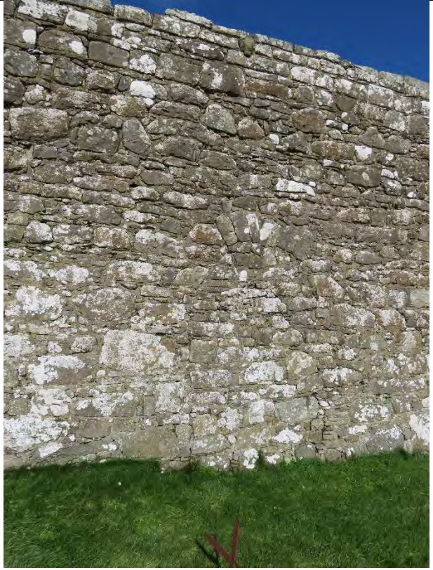
Image showing corresponding door opening to the external wall.
