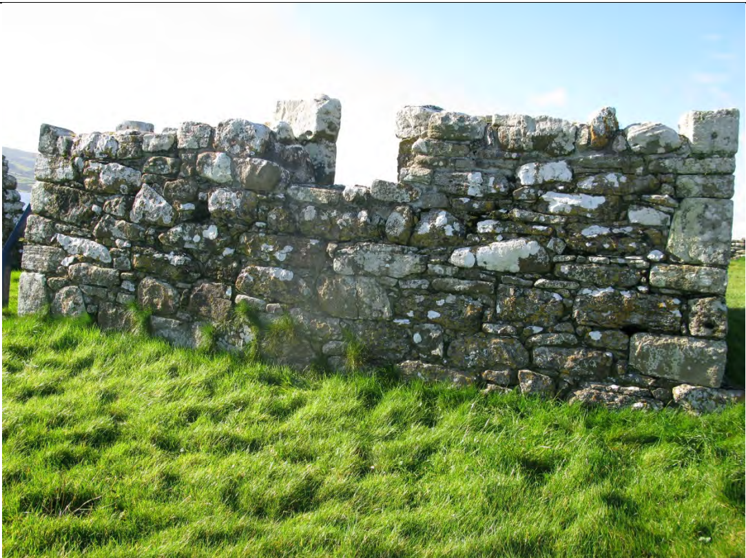
Image showing east elevation to St Brigid's Church which was reconstructed in the 1970s. Note grass growth in the lower joints.
