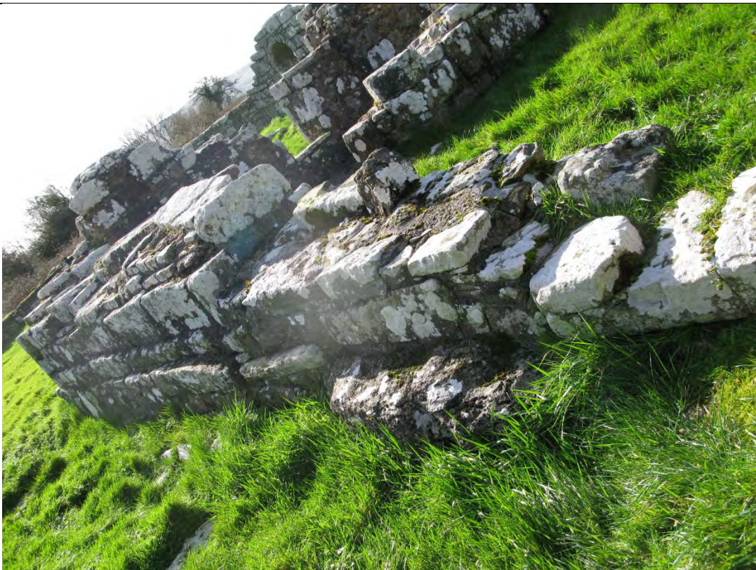
Image showing west wall to Teampall na bhFear nGonta. Loss of flashing to skyward surface.
