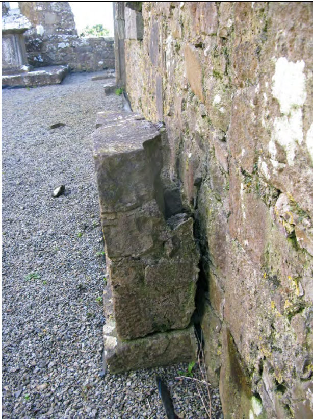
Image showing carved stone to south wall.
