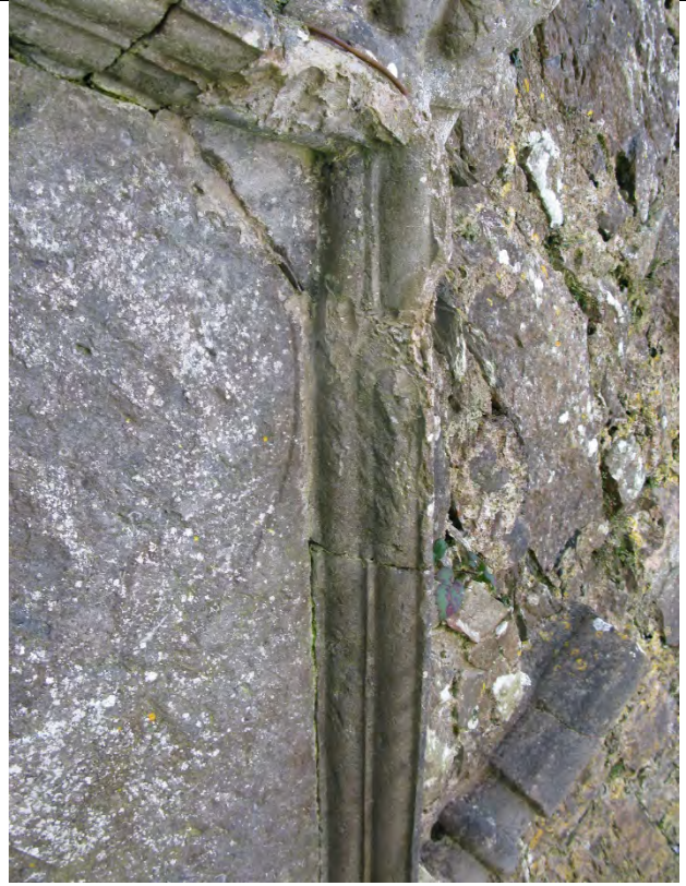
Detail showing chipped and damaged stone with poor repairs.
