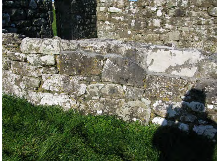
Detail showing cementitious flashing and pointing to south elevation St Brigid's Church.
