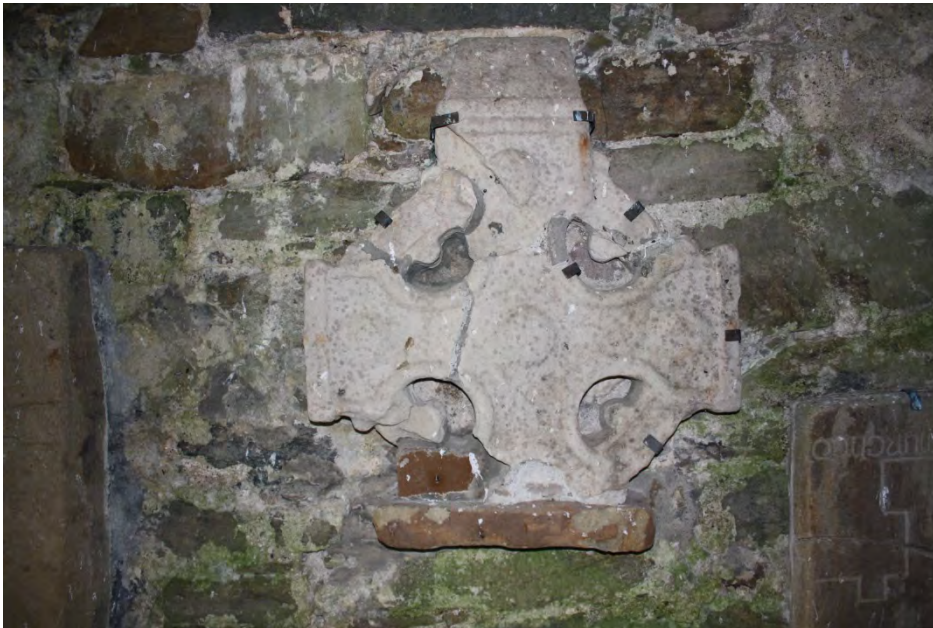
Fig. 81: Wheeled cross-head, south wall of St Caimín’s Church, note breaks, metal supports, and cementitious material (Photo: C. O’Leary)
