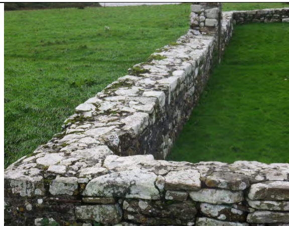
Image showing south wall to St Brigid's enclosure. Note the extensive vegetative growth to the skyward surface of the wall.
