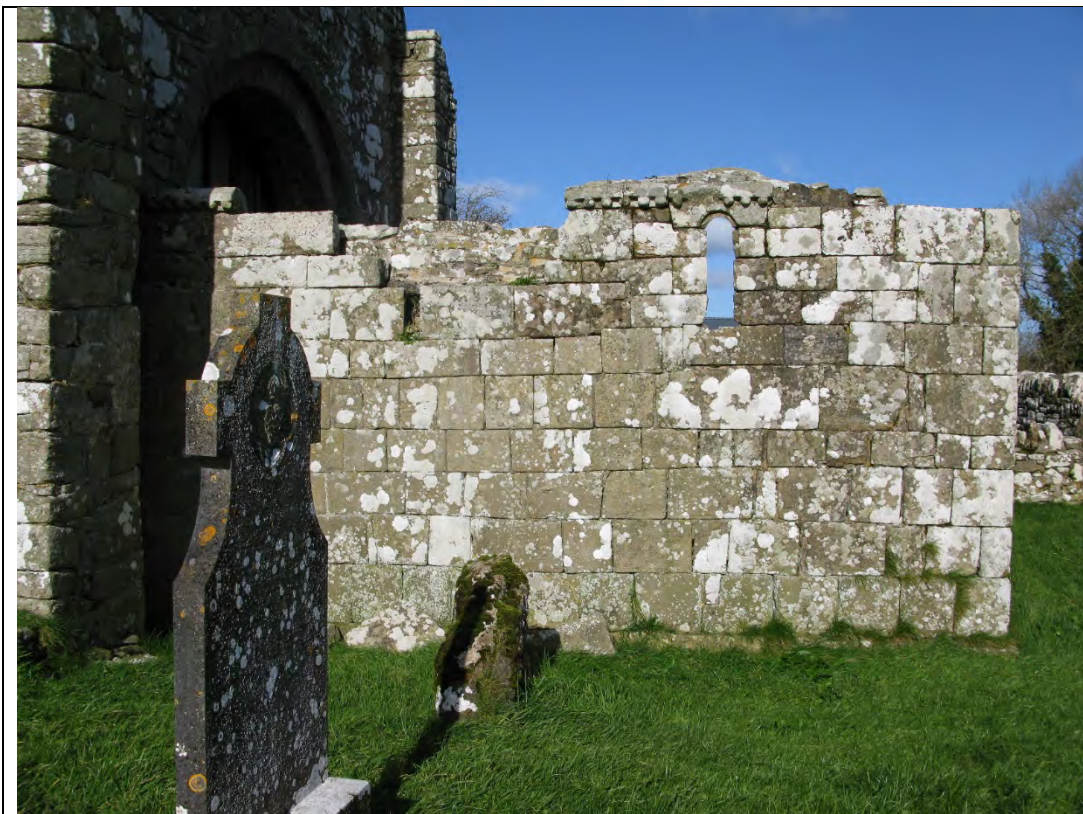
Image showing south elevation to chancel. Note open joints throughout, failure of flashing, ashlar missing (located at base) and vegetation to wall top and grass growing in open joints.
