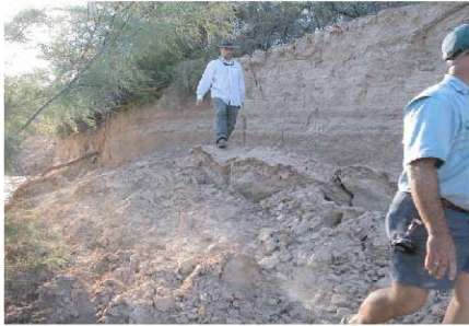
Figure B.9.1. Collapsing channel banks in ephemeral channel approximately one half mile above headwaters of the North Fork and downstream from Arrow Canyon.
