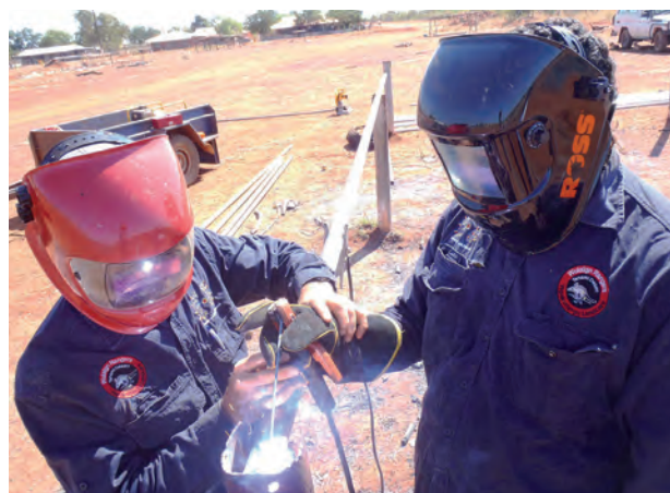
Rangers receiving welding training as part of repair to horseyards near Lajamanu
