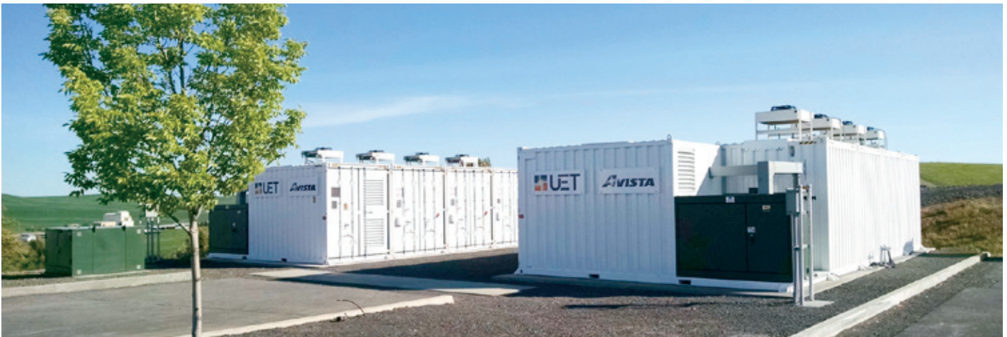
A 1-megawatt/4-megawatt-hour vanadium flow battery owned by Avista Utilities in Pullman, Washington.
