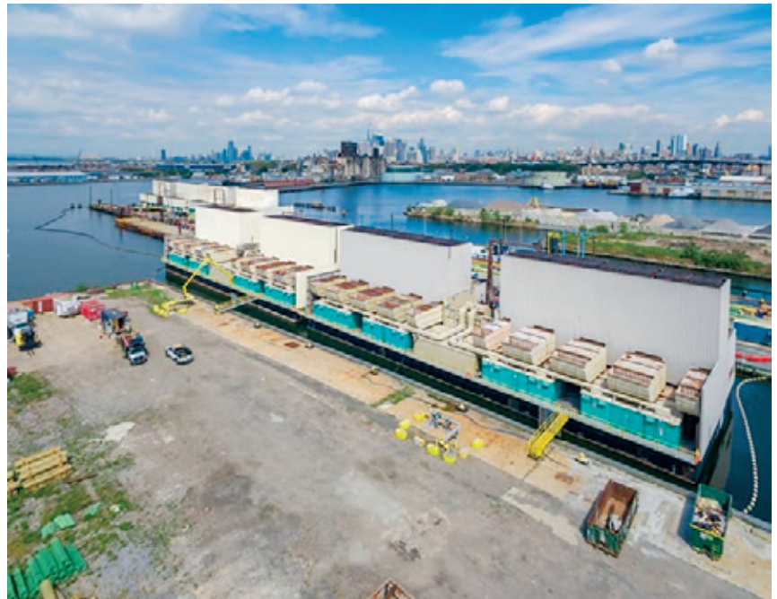
352-megawatt Narrows Peaker Plant in Sunset Park (ArcLight Capital Holdings LLC/AGC)
