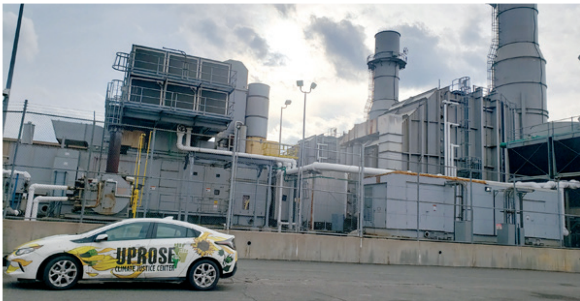
94-megawatt Joseph Seymour Peaker Plant (NYPA)
