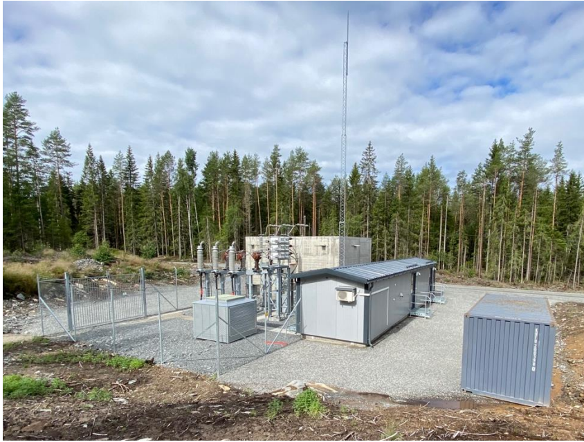
Figur 12 Transformatorstation i Marker Vindpark, Norge
