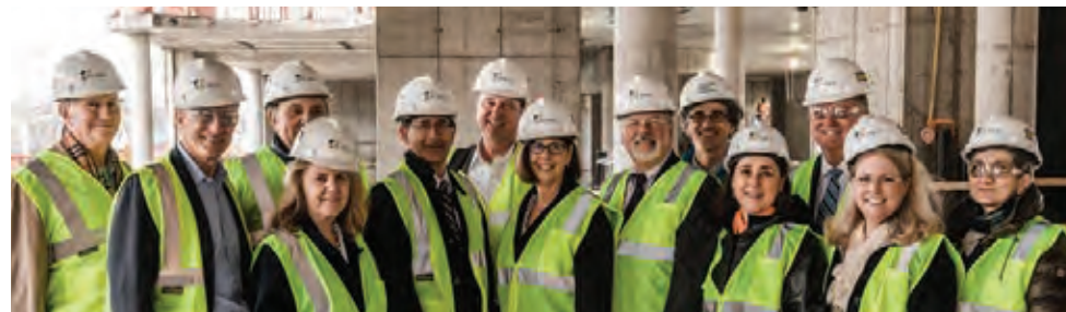
Members of the Tepper School's Business Board of Advisors tour the Tepper Quad construction site.
