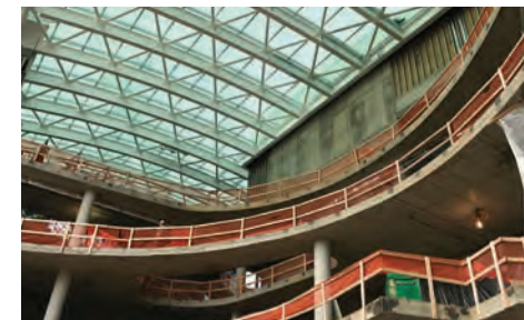
This fall, the new Tepper Quad building exterior was completed, enclosing the building in glass and brick.
