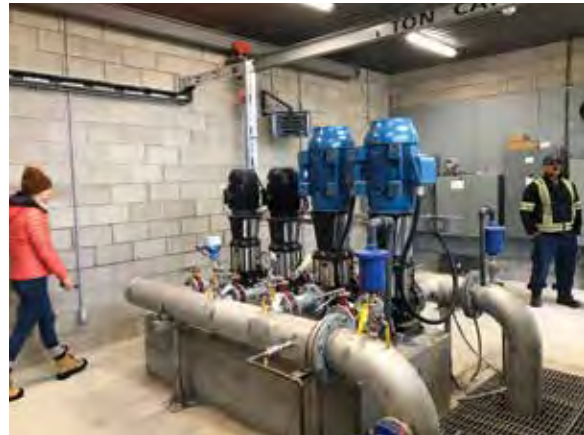
Visit by CIMA+ to Mistissini Booster Station
