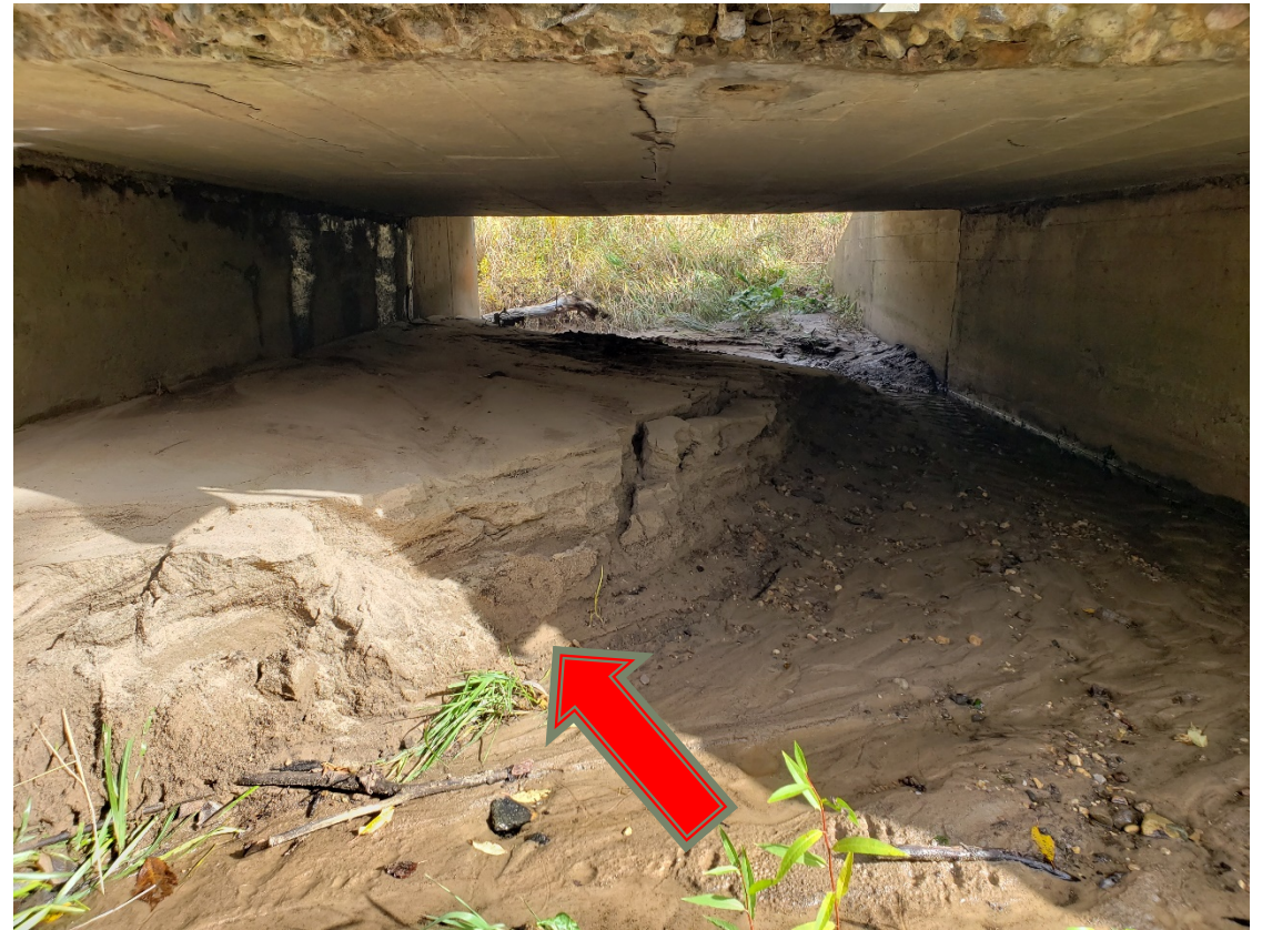
View of Wilson Creek flowing under the bridge looking upstream. Note sediment collection on the left.
