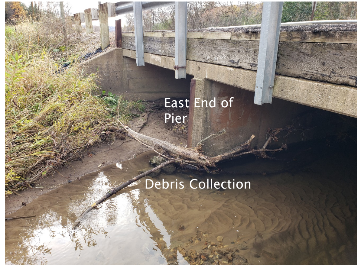
This photo shows the tendency for debris and sediment to collect near the pier.
