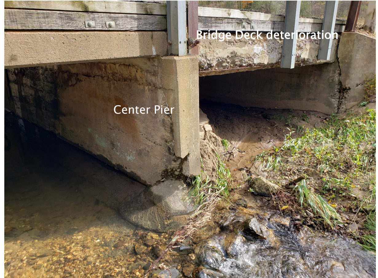
View of the deteriorating center pier and bridge deck. Salts applied during the winter escalate the deterioration of the bridge deck.
