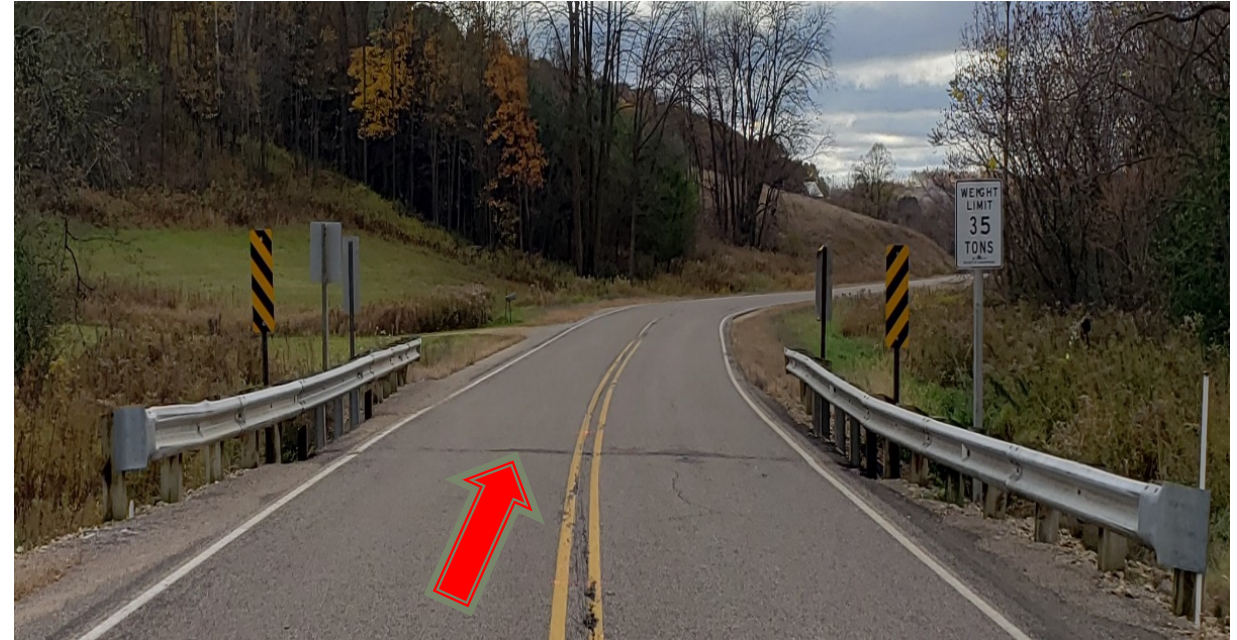
Arrow shows ledge between the bridge and adjoining roadway caused by settlement of the road in front of the abutments (looking southeast).
