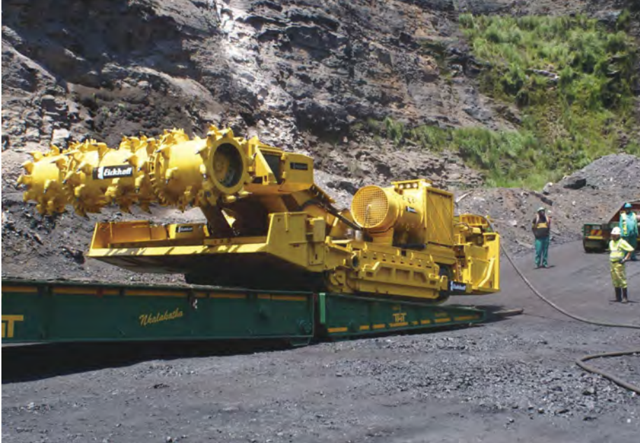
A new Eickhoff CM2 is being offloaded in the box cut at Halfgewonnen.
