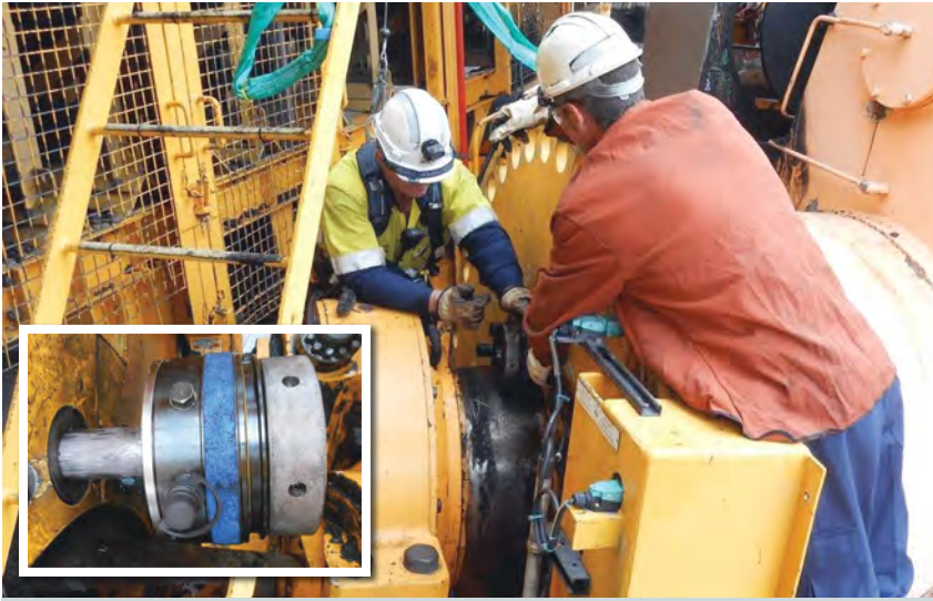
Technicians use a custom hydraulic tensioner (inset) to remove 3-m-long studs in a confined space.
