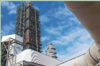
Sixteen-foot diameter ductwork takes flue gas from the coal plant to the carbon capture facility where the CO 2 is removed from the flue gas. (Photo: NRG)
