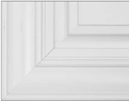
Example of door front joint separation
