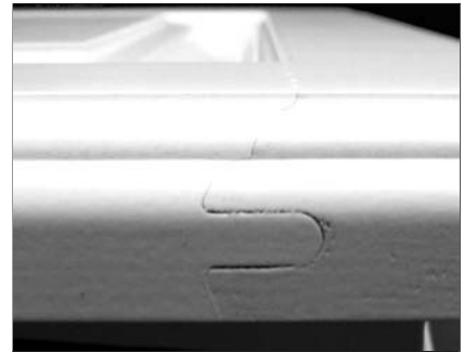
Example of door end joint separation
