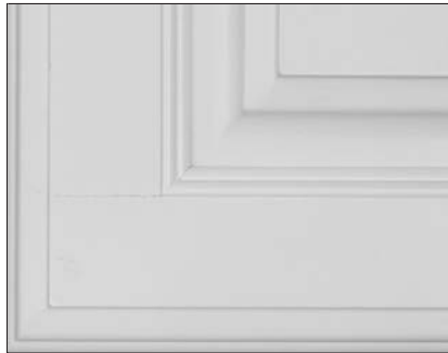
Example of door front joint separation
