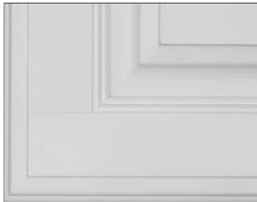
Example of front joint separation
