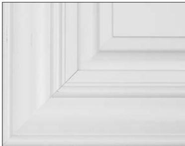
Example of front joint separation
