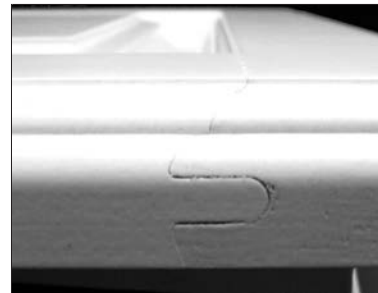
Example of end joint separation
