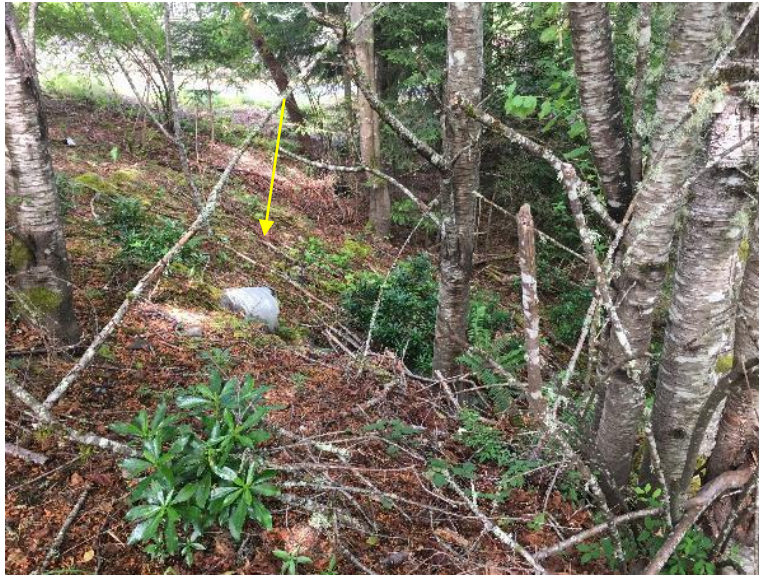
Photograph 12. Steel corrugated culvert adjacent to Zapata Place to the north of the Site.
