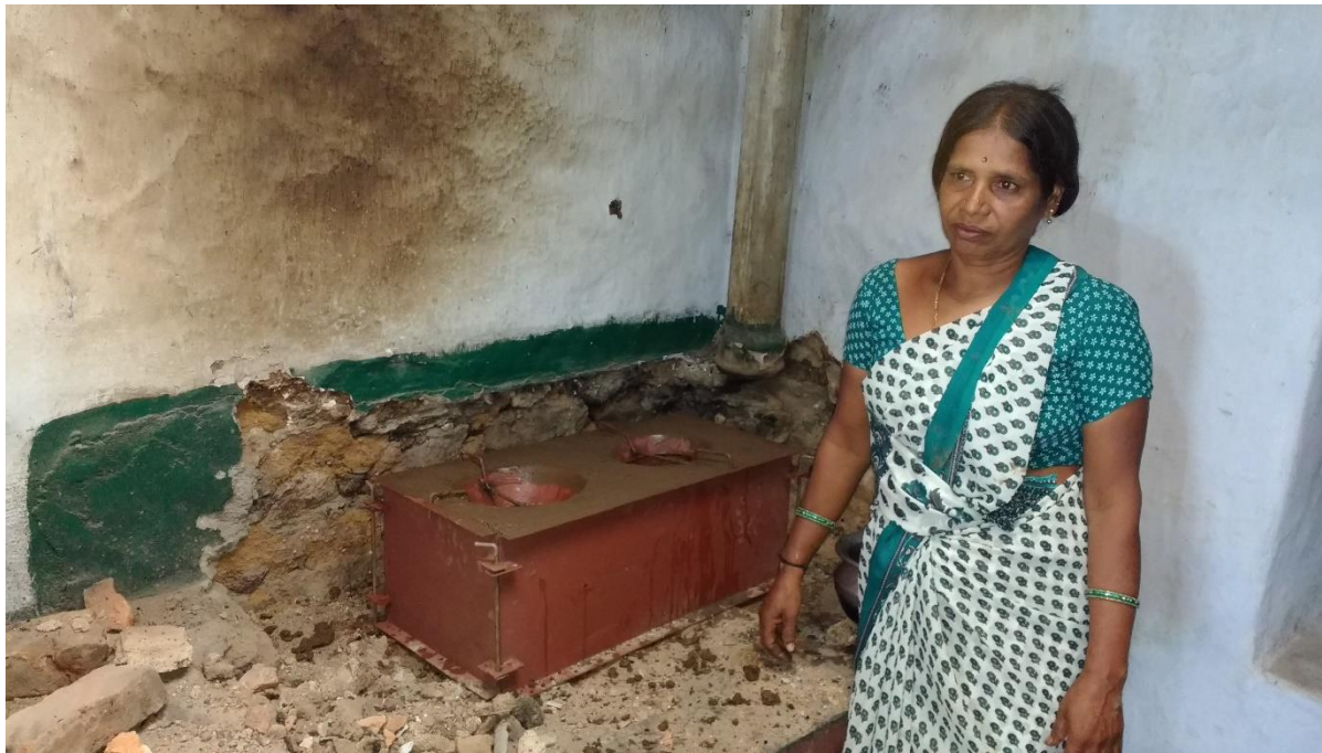
Image 4. Installation of the energy-efficient stove by Sustaintech/TIDE, Bangalore at Munnar, Kerala
