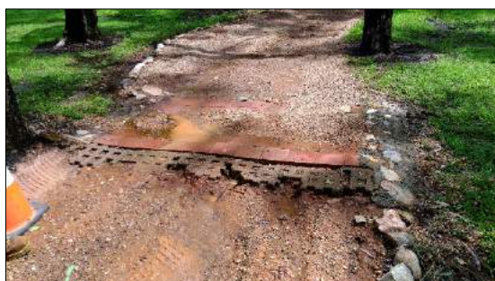
Erosion of Primary Path
