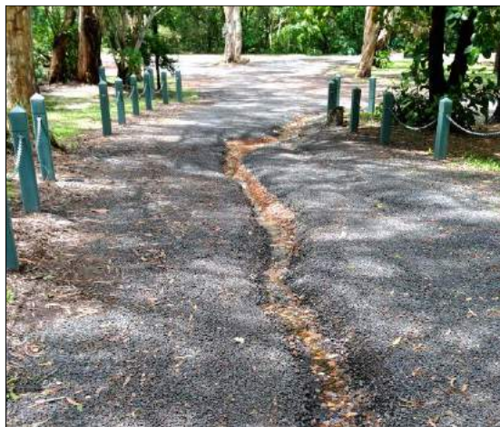
Runoff damage to the Entrance Driveway
