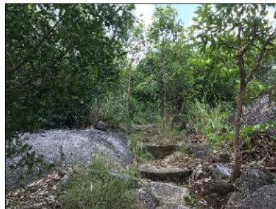
Weed infested damaged Track to CTB
