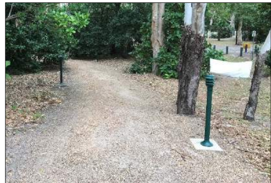
Access path from the carpark to NPH. Note dated bollard light style, which needs upgrading
