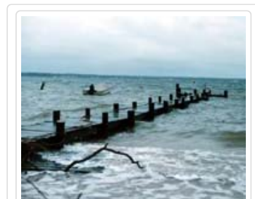
High tide combined with a storm threaten a pier. (Photo: Mary Hollinger)
